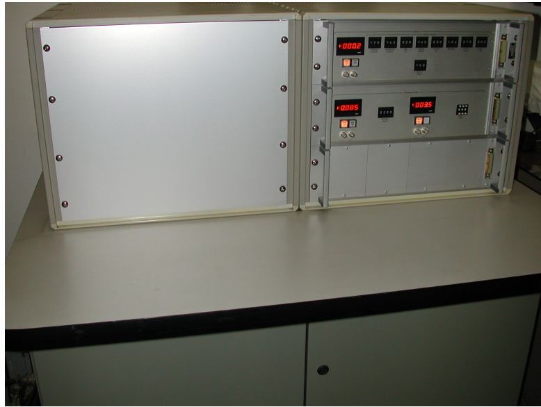
Figure 3.2: Electronic control unit of the MVT equipment.
