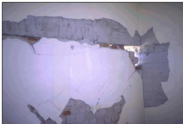
Figure 6.35 Severely damaged infill wall between columns G12 and F12 at the first story
