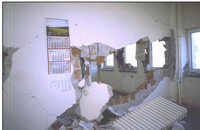
Figure 6.32 Collapsed infill wall between columns D10 and E10 at the first story
