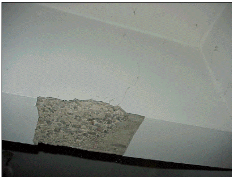
Figure 6.60 Diagonal crack about 60 cm away from the end of beam spanning between E5 and E6 at the ground story
