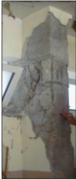
Figure 6.12 Failed column D10 at the ground story
