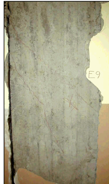
Figure 6.29 Diagonal cracks in column E9 at the first story
