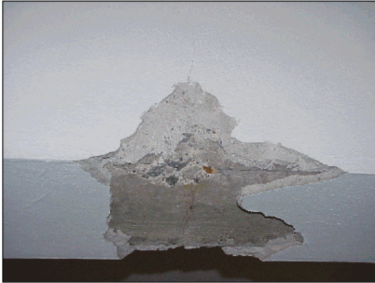
Figure 6.67 Flexural crack, about 50 cm away from the left end of the beam spanning between B7 and B8 at the ground story
