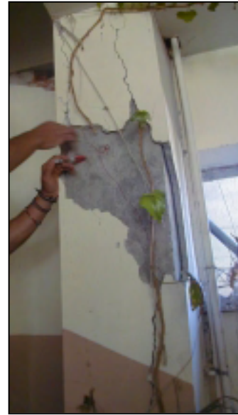
Figure 6.10 Diagonal crack in column D9 at the ground story
