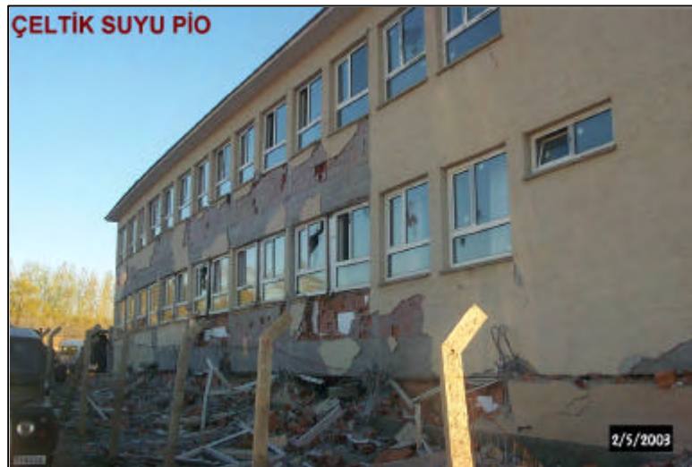
(b) School building (Fully collapse of ground story)
