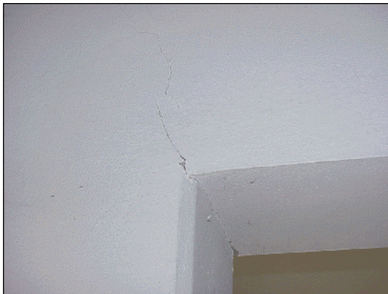
Figure 6.62 Flexural crack at the end of the beam spanning between A6 and B6 at the ground story
