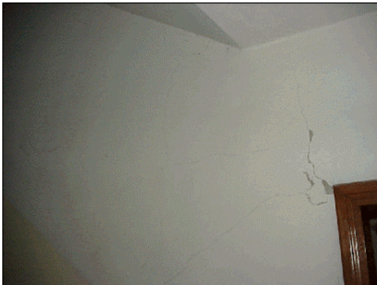
Figure 6.64 Flexural crack at the end of the beam spanning between B9 and C9, where it spans into the shear wall P2, at the ground story
