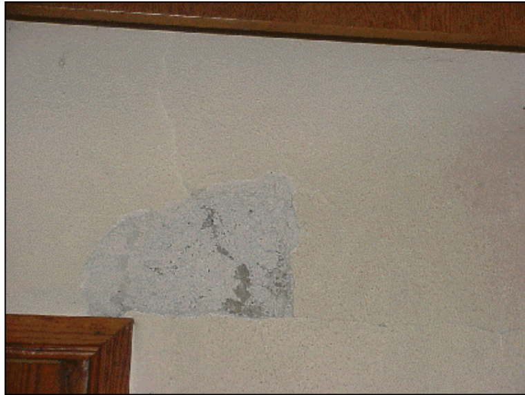
Figure 6.65 Flexural crack, about 80 cm away from the end of the beam spanning between A8 and A11 at the ground story
