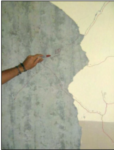
Figure 6.16 Diagonal cracks in column E10 at the ground story
