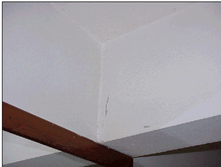
Figure 6.68 Flexural crack at the right end of the beam spanning between B7 and B8 at the ground story
