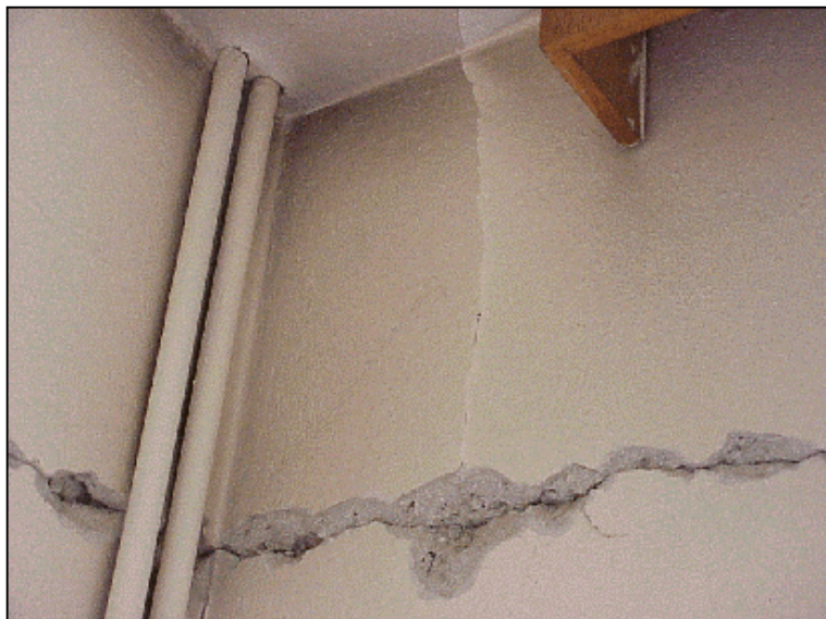
Figure 6.66 Flexural crack, about 30 cm away from the end of the beam spanning between D12 and F12 at the ground story
