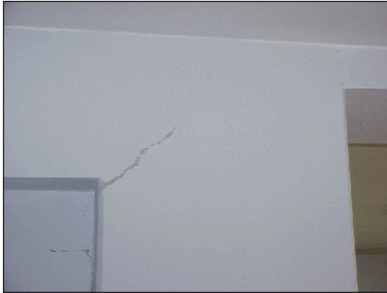
Figure 6.61 Diagonal crack in the beam spanning between B2 and C2 at the ground story
