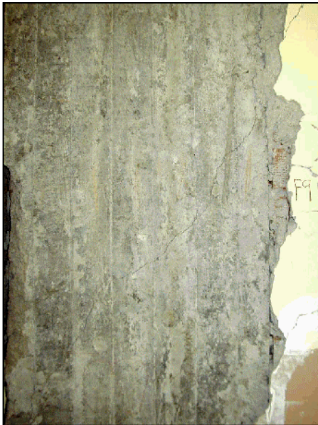
Figure 6.37 Diagonal crack in column F9 at the second story
