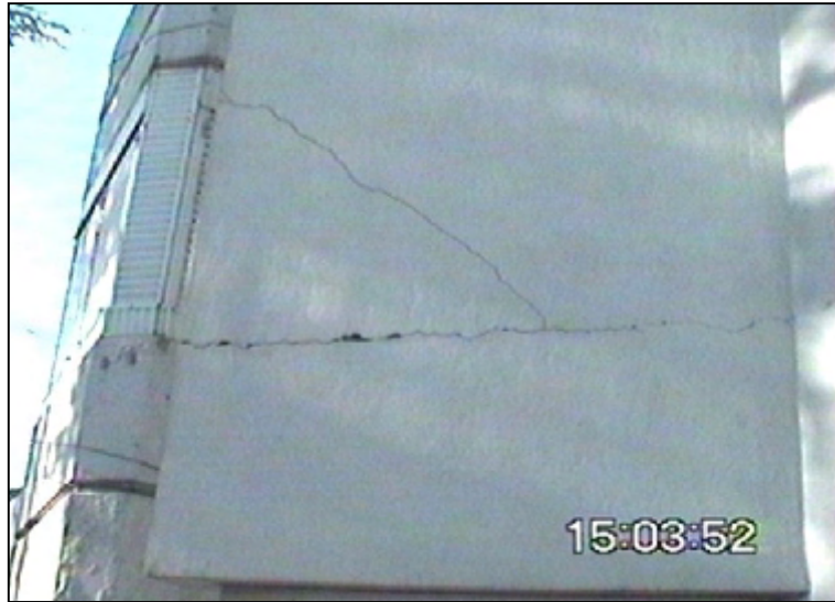
Figure 6.57 Cracking on of the second story exterior infill walls at the right-side (south) of the building
