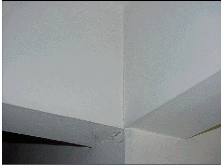
Figure 6.63 Flexural crack at the end of the beam spanning between B8 and C8 at the ground story
