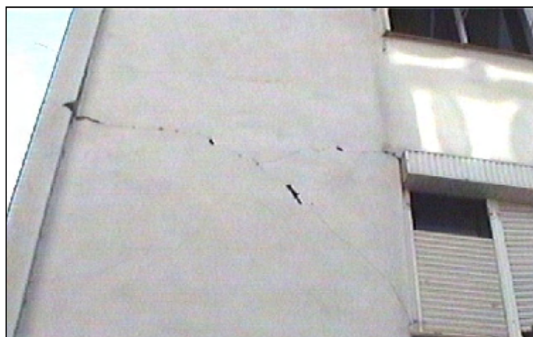
Figure 6.56 Cracking on the second story exterior infill wall at the back side (east-west direction) of the building
