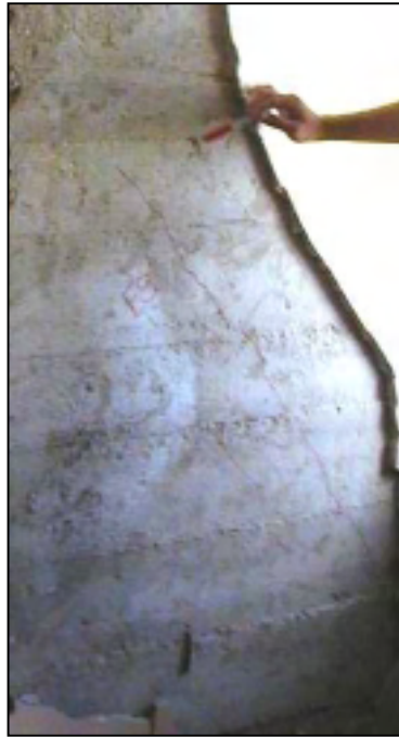
Figure 6.19 Diagonal crack in column F8 at the ground story
