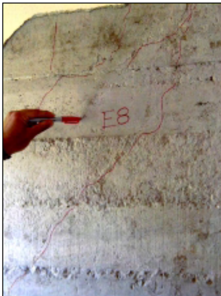
Figure 6.14 Shear cracks in column E8 at the ground story
