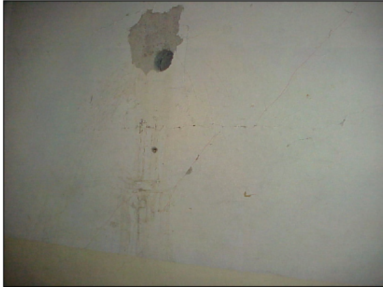
Figure 6.59 Diagonal cracks on the web portion of the shear wall P2 and horizontal crack along the slab level of the ground story
