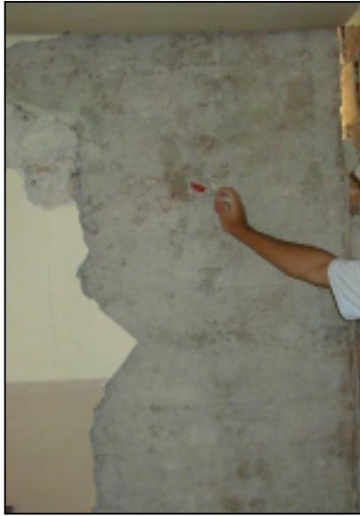
Figure 6.9 Diagonal crack in column D8 at the ground story
