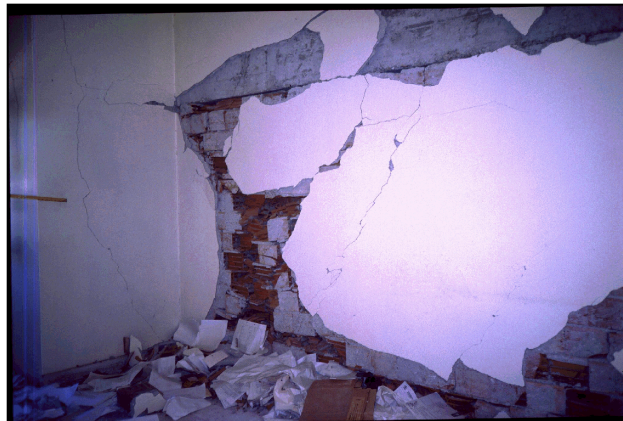
Figure 6.34 Severely damaged infill wall between columns D12 and F12 at the first story
