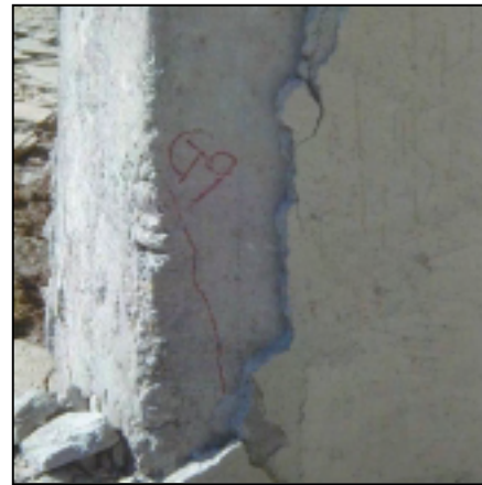
Figure 6.24 Diagonal crack in column G9 at the ground story
