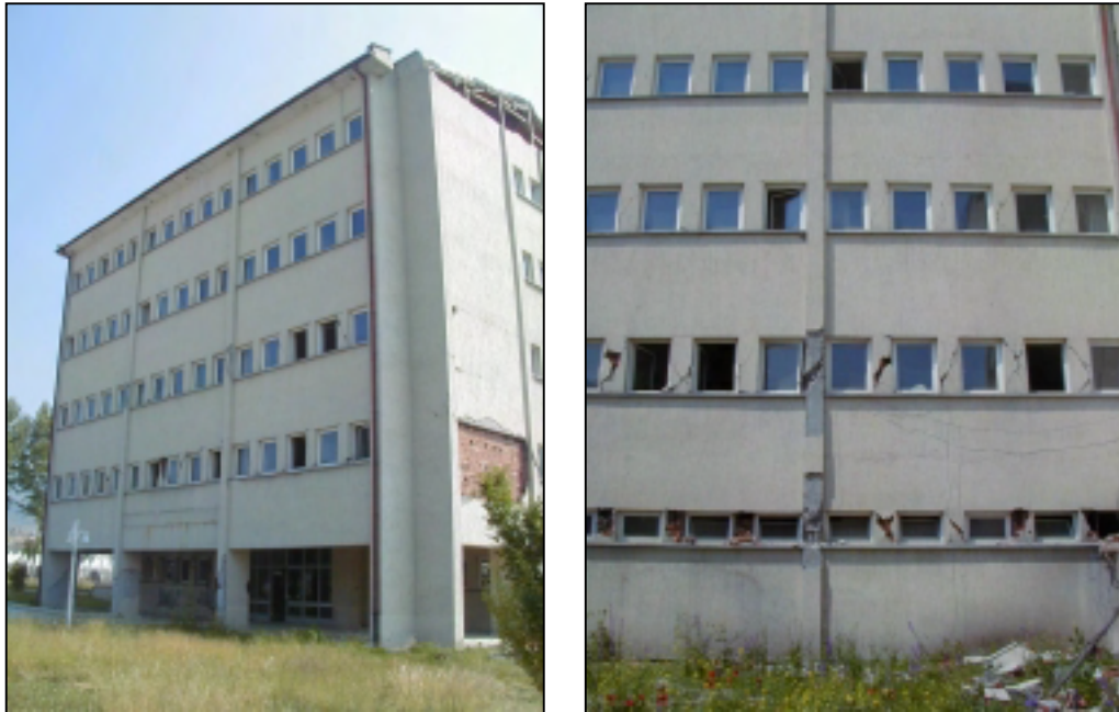
Figure 6.5 Damage state of the case study building
