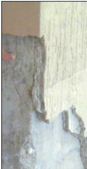
Figure 6.21 Crack observed in column F10 at the ground story
