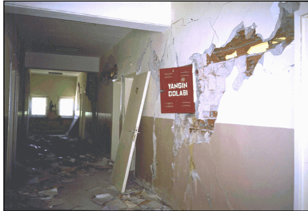
Figure 6.33 Severely damaged infill wall between columns F9 and F7 at the first story
