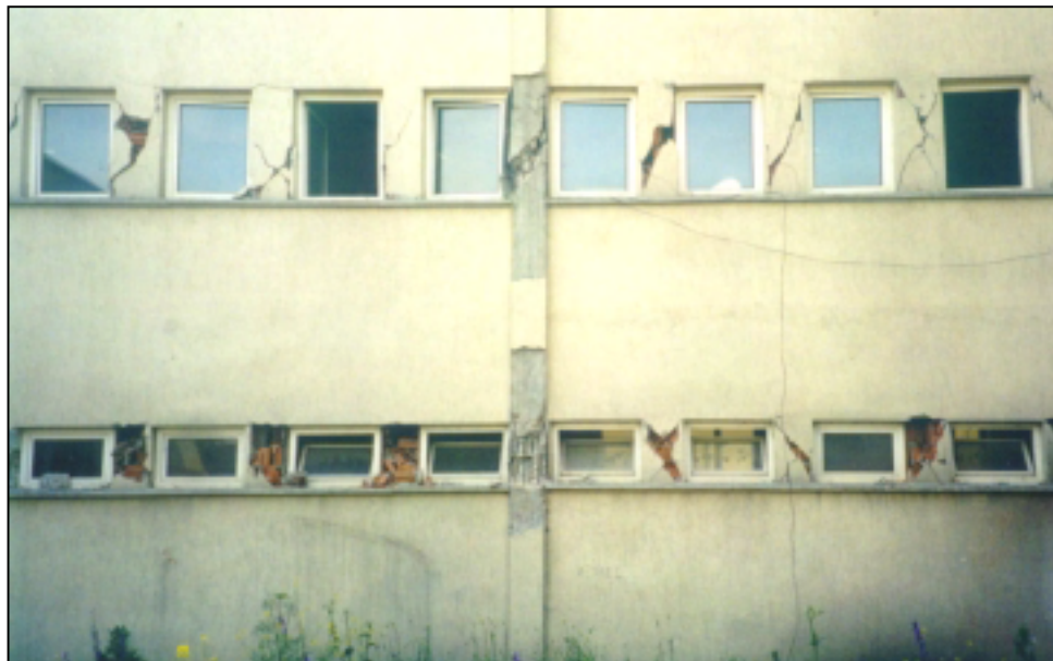
Figure 6.18 Cracked masonry infill walls between D9 and D12 columns at the ground and first story levels (rear elevation)
