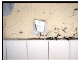
Figures 5.17-18-19 Items damaged during use (building 'C')
