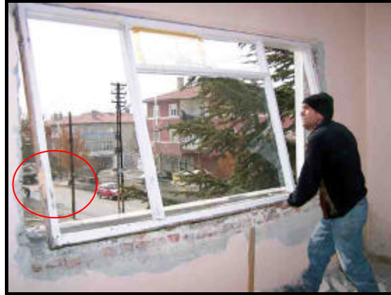
Figure 5.29 The window was damaged due to the use of wooden anchors fixing it to the walls (building C)
