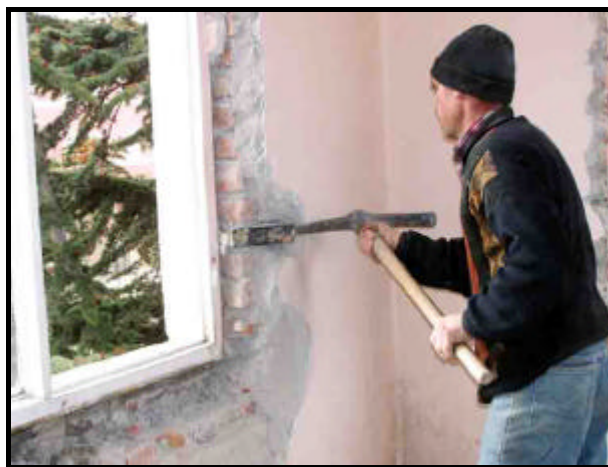
Figure 5.28 Recovery of wooden anchors, which were used to fix the window to the walls (building C)
