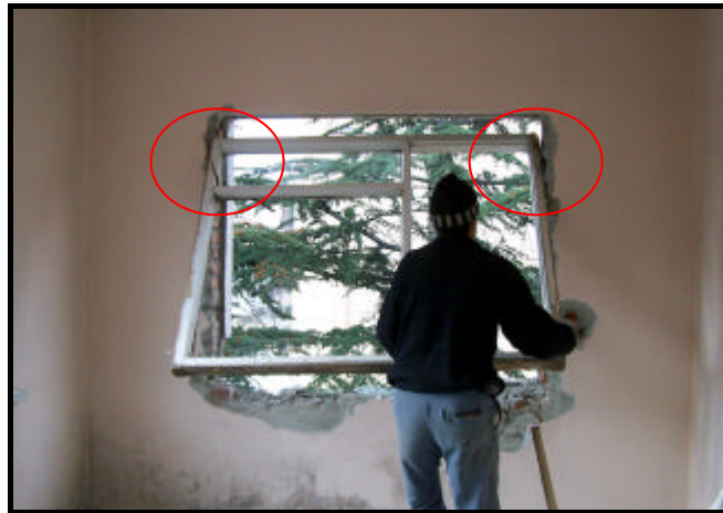
Figure 5.31 The window was wasted due to damage caused by lack of worker experience (building C)
