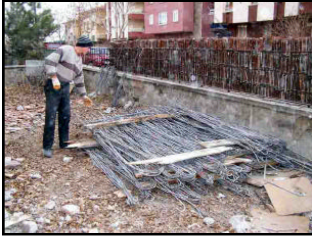
Figure 5.13 Rebar recovered from building C
