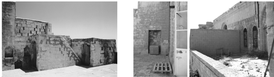
Fig. 4.13 The locked door of the staircase to prevent passage between floors, Gözü House (photograph: Mert Kayasü).
