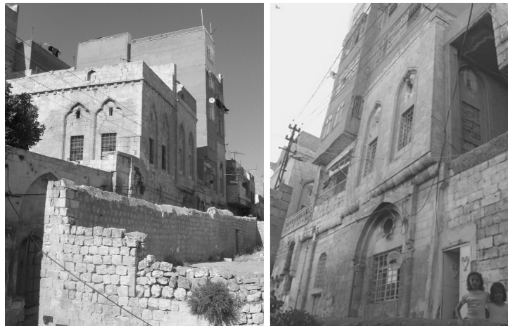
Fig 2.5 A hybrid building with a reinforced concrete addition to a historical masonry building. Notice the style difference between the two, how the addition exceeds the height of the house next to it and avoids the view of the house behind it (photograph 1: Mert Kayasü, photograph 2: Aydan Balamir).
