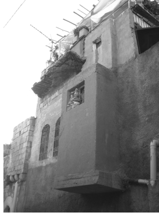
Fig 2.7 An example of a minor intervention: an addition of a toilet to the structure (photograph: Mert Kayasü).
