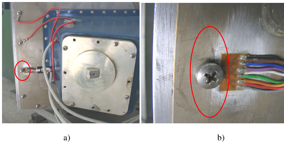
Figure 6.17: Front view of the crack location, a) Wide view, b) Closer view.
