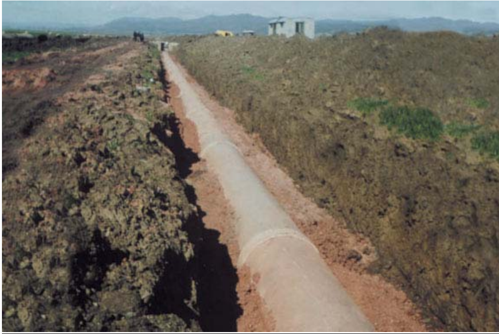
Figure 3.8 GRP Water Transmission Line ( www.superlit.com )
