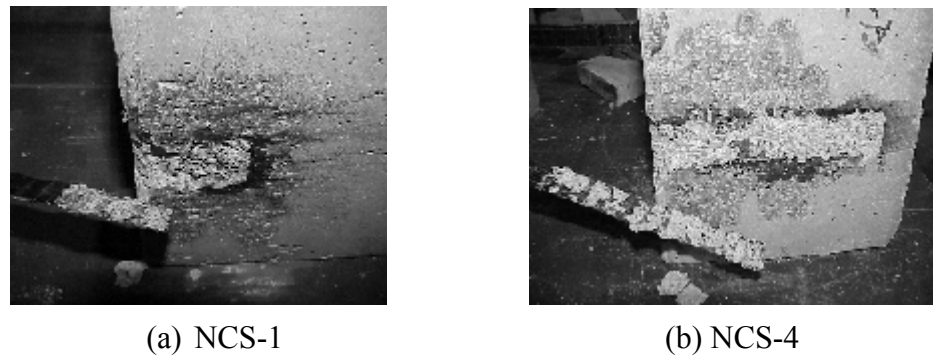
Figure 2.16 Pictures of Debonding in Concrete
