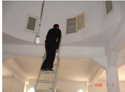
Figure 5.66: Balat al-Shoha'da Mosque, Poor Design, Poor Workmanship
