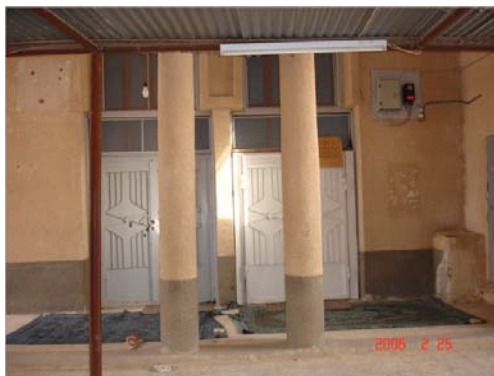
Figure 5.82: Bab al-Ray'yan Mosque, Unsuitable location of Columns
