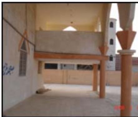
Figure 5.39: Ghazwat Ohed Mosque, Dispensable Spaces, Poor Workmanship
