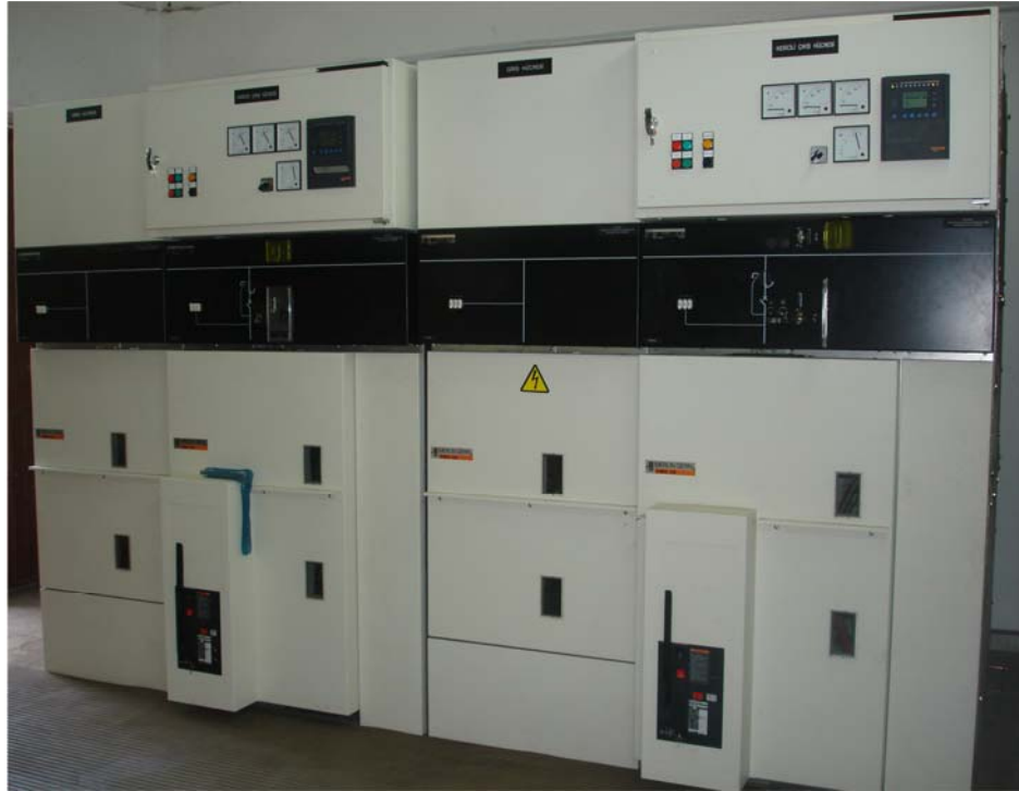
Figure 3.17 6.3kV Switchgear Cubicles
