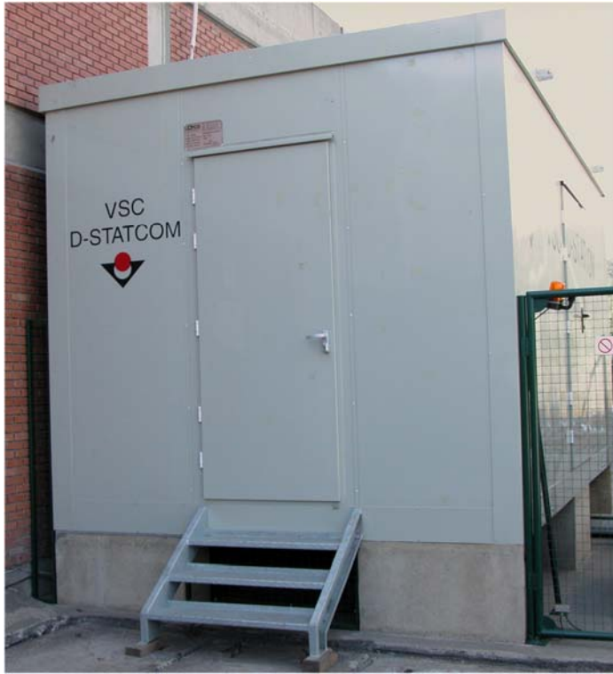
Figure 3.18 STATCOM LV Container
