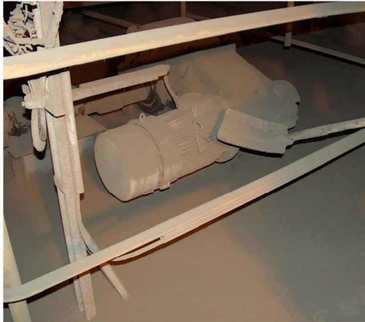
Figure 3.4 Belt Conveyor Motors with Excessive Coal Dust
