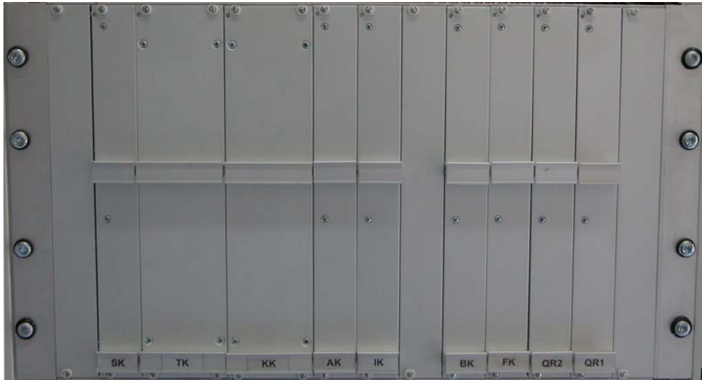
Figure 3.60 Control System Hardware
