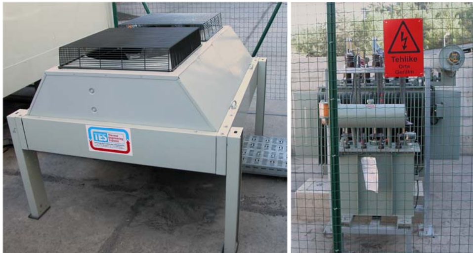
Figure 3.19 HX Unit and Coupling Transformer
