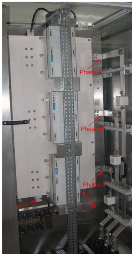
Figure 4.4 Implemented Power Stage of VSC
