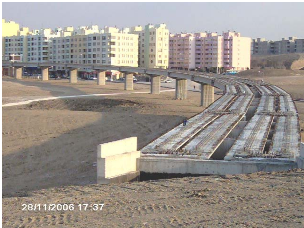
Figure 3.4 Ankara Rail Transit System / Stage 3 Works Construction Part Passing Away from Batıkent
