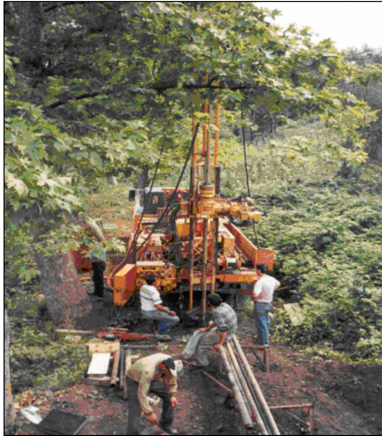
Figure 2.5 Exploratory boring drilled for SPT performance on field during a site investigation Black Sea Region / TURKEY
