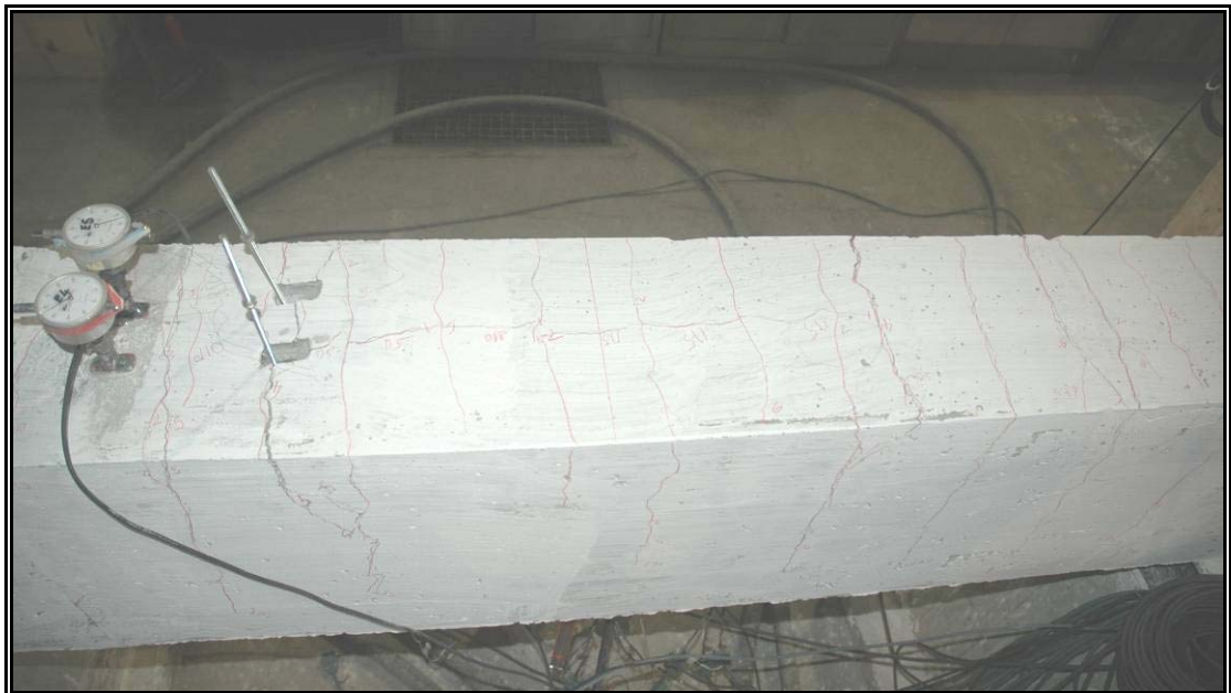
Figure 4.23 TS16 splice region after test.
