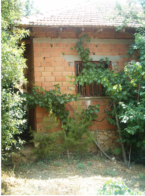
Figure 4.12 Hybrid structure at Gümüşkol Village (rubble stone foundation and cellular brick wall are laid using clay mortar, lintel above window and roof slab are reinforced concrete)
