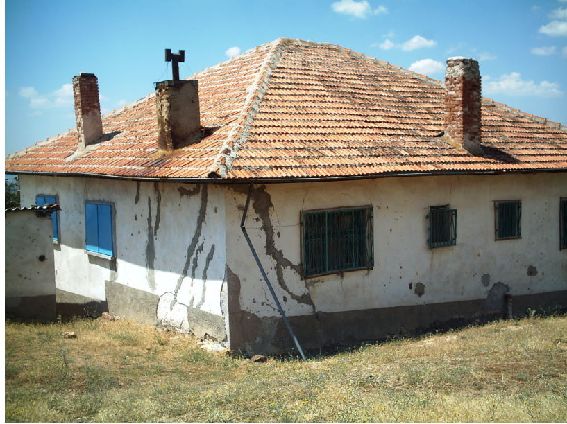
Figure 4.10 The repaired tension cracks at the corner of the building formed previously due to differential ground settlement or weak foundation at Gümüşkol Village
