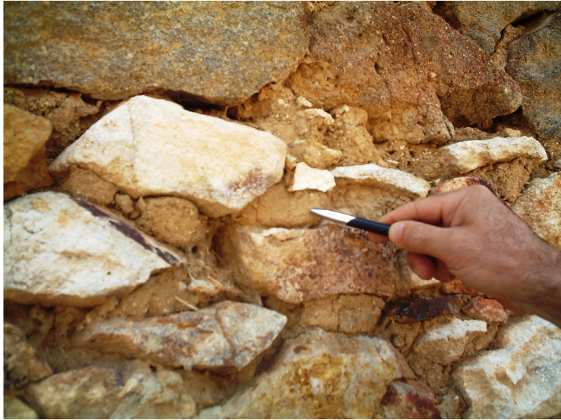
Figure 4.9 Close in view of clay mortar at the bare wall of rubble stone building at Gümüşkol Village
