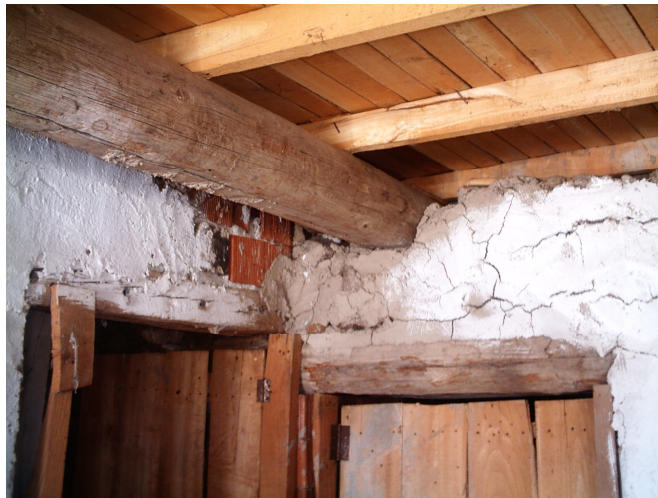
Figure 4.15 House at Micanlar District (deflection of wood beam, resting on interior door lintel instead of a column, contributed to the development of shear crack at the wall intersection in Figure 4.14)
