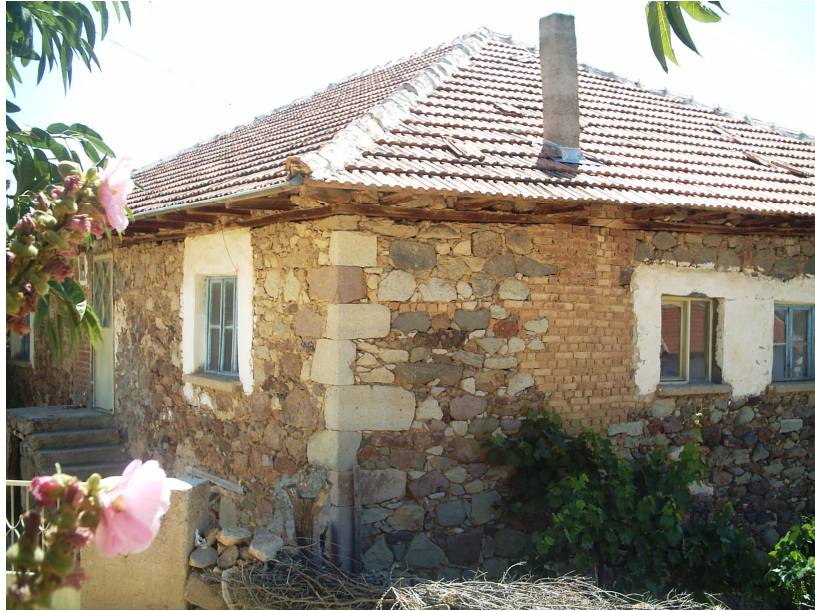
Figure 4.8 Clay mortared hybrid (undressed and dressed stones and solid bricks) structure at Gümüşkol Village
