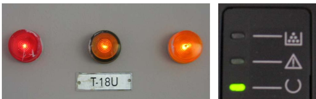
Figure 2-6: Power On Lights
