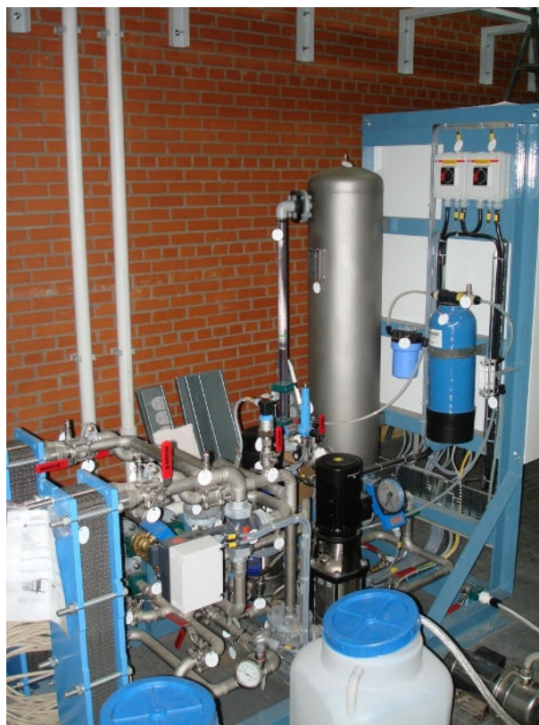
Figure 4.25 Water Cooling System of the ETT Stacks Used for TCR System
