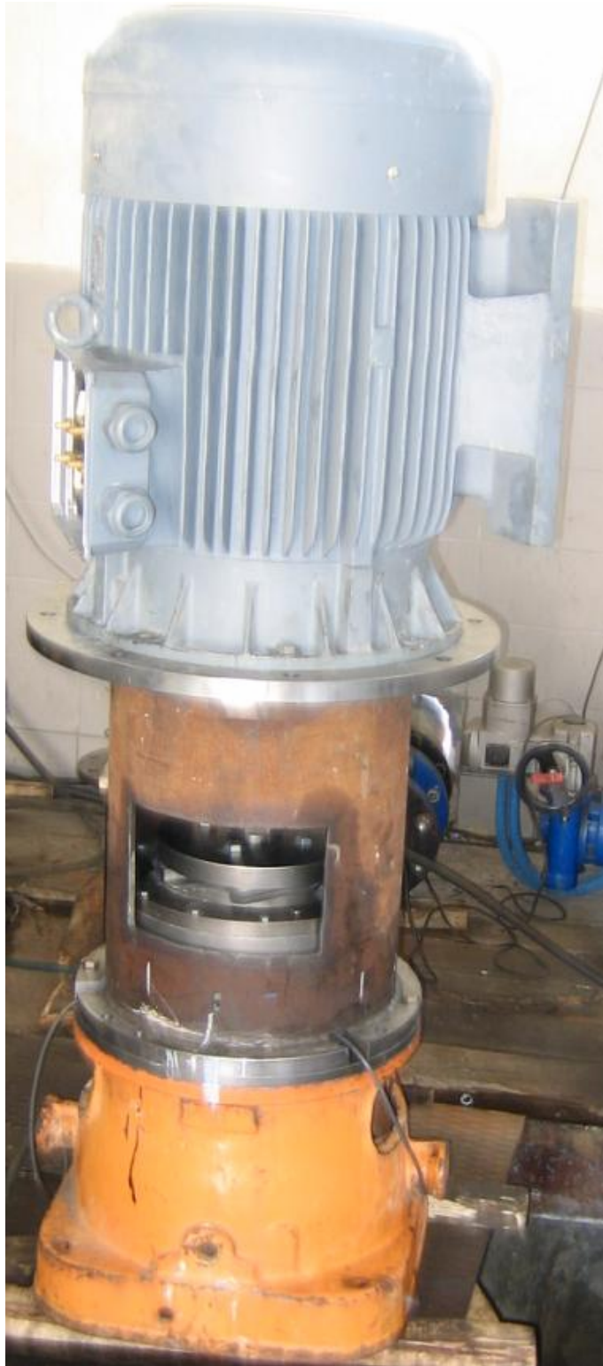
Figure A.6 Pump assembly and motor
