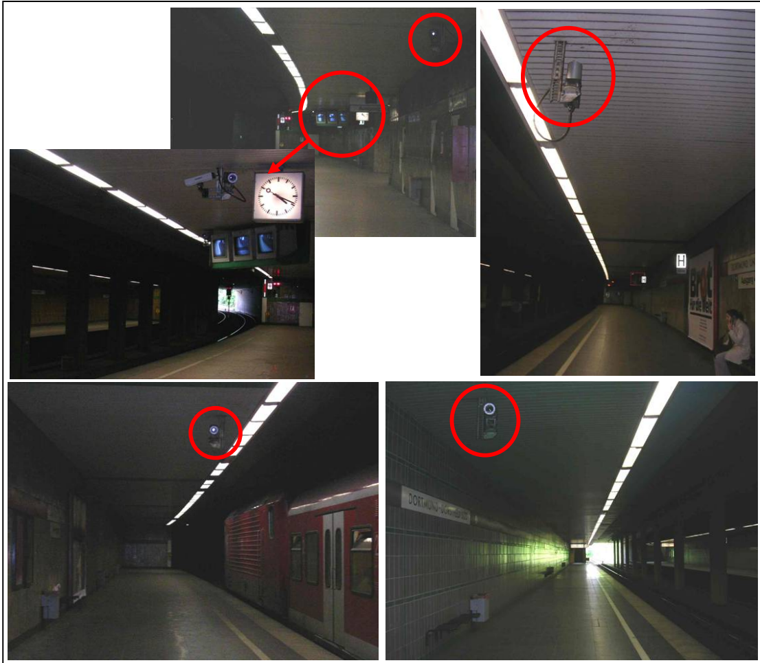
Figure 6.7 Examples for CCTV in public spaces such as train stations from a German city Note: For better visibility the installed systems are encircled
