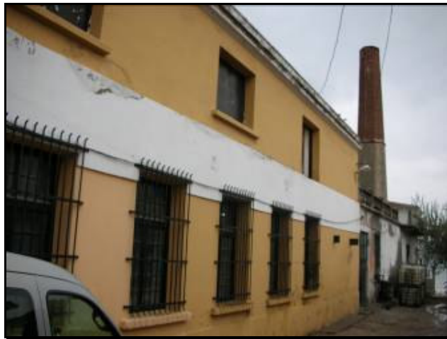
Plate 4.29: Hexagonal chimney decorated with the cross symbol, unique in Ayvalık. Usually conic chimneys were built with no decorations, Building # 16.
