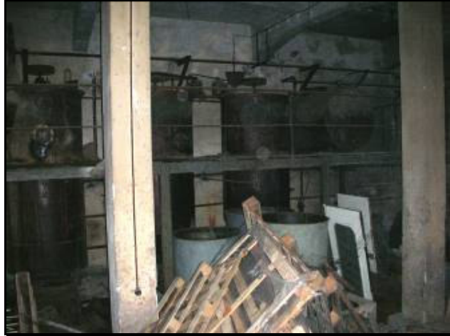
Plate 4.26: Steam boilers, Building # 16.
