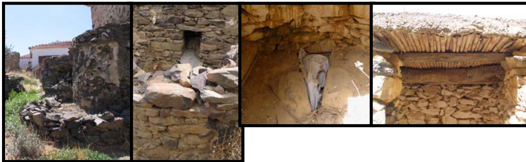
Figure 49 The circular toilet spaces are surrounded by a shorter stone wall which edges the in between space that is full with earth
