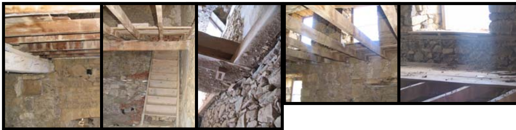
Figure 57 10 to 12 centimeters difference in the width of the ground and first floor walls is utilized as a base for the perpendicular timber beams of the floor of the first storey
