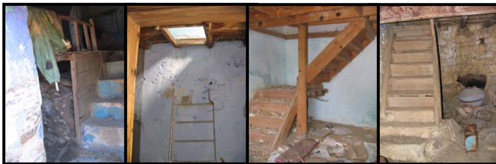
Figure 69 Only stone stairs in one storey houses/ Portable timber or iron stairs in double storey houses/ fixed timber stairs/ Timber stairs fixed on stone steps
