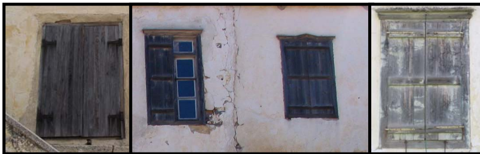
Figure 67 Two kinds of shutters; fitting to the opening and framing the opening
