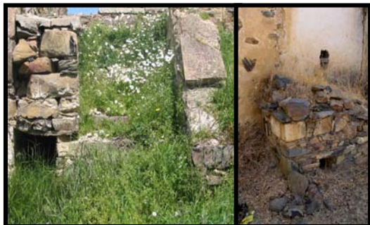
Figure 47 Coops are attached to the front façade and accompanied with folluk holes or fitted to the space under outdoor stair of houses
