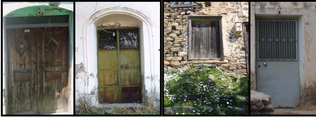
Figure 65 No. 29 and no. 112 are double winged doors with an arched door opening and no. 85 and no. 141 are single winged doors with flat door opening. No. 112 and no. 141 are metal doors with glass and metal balustrade, which is the most common intervention type on old timber doors
