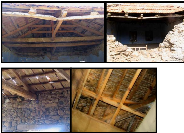
Figure 62 Pitched roof is either decked by timber planks over beams and the structure is exposed or it is decked by straw, the traditional material of flat roofs, and covered by timber planks as the ceiling material
