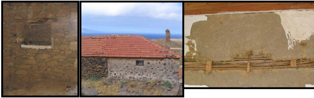
Figure 58 Inside and outside of an exterior wall is constructed with same stone and technique. The partition walls are applied in the traditional technique
