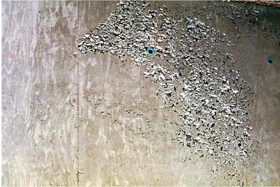
Figure 1.11 Honeycombing in a concrete *
