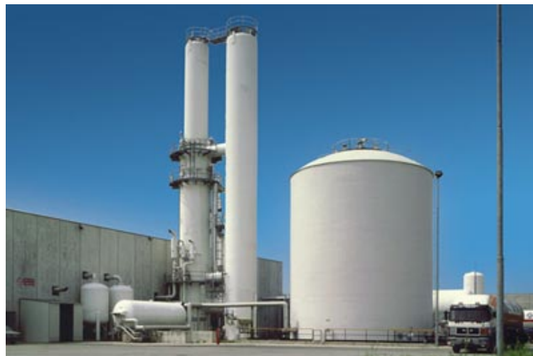
Figure 5.9. Cryogenic oxygen plant (www.grasus.com)
