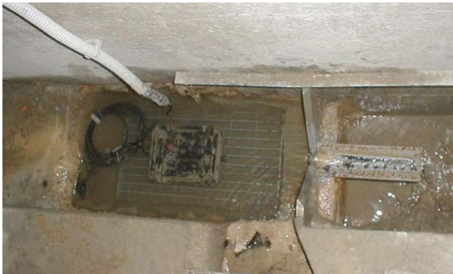
Figure 4.6. Typical installation of V-Notch weir with pressure transducer unit (SIS, 2008)
