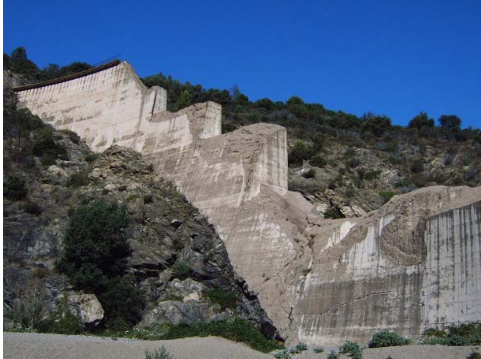
Figure 1.2. Remaining right abutment of Malpasset Dam
