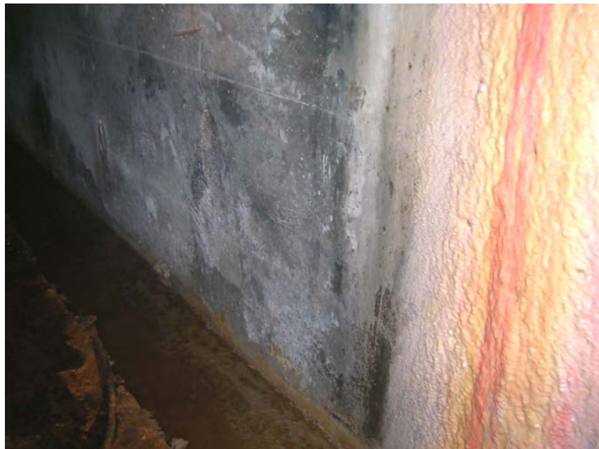
Figure 5.2. Accumulation of minerals at the 195.50 m gallery of Cindere Dam during initial filling
