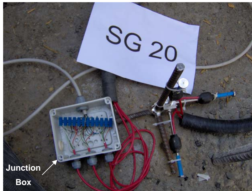
Figure 4.2. 3-D rectangular strain gauge rosette installation at the upstream face of Cindere Dam
