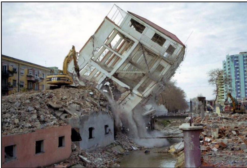
Figure13: Demolition over the Lana River of one the highest buildings erected along the river, 2003, (Source: http://www.shqiperia.com , http://www.shqiperia.com/galeria/main.php?g2_itemId=29193 , accessed on 11/06/2008)
