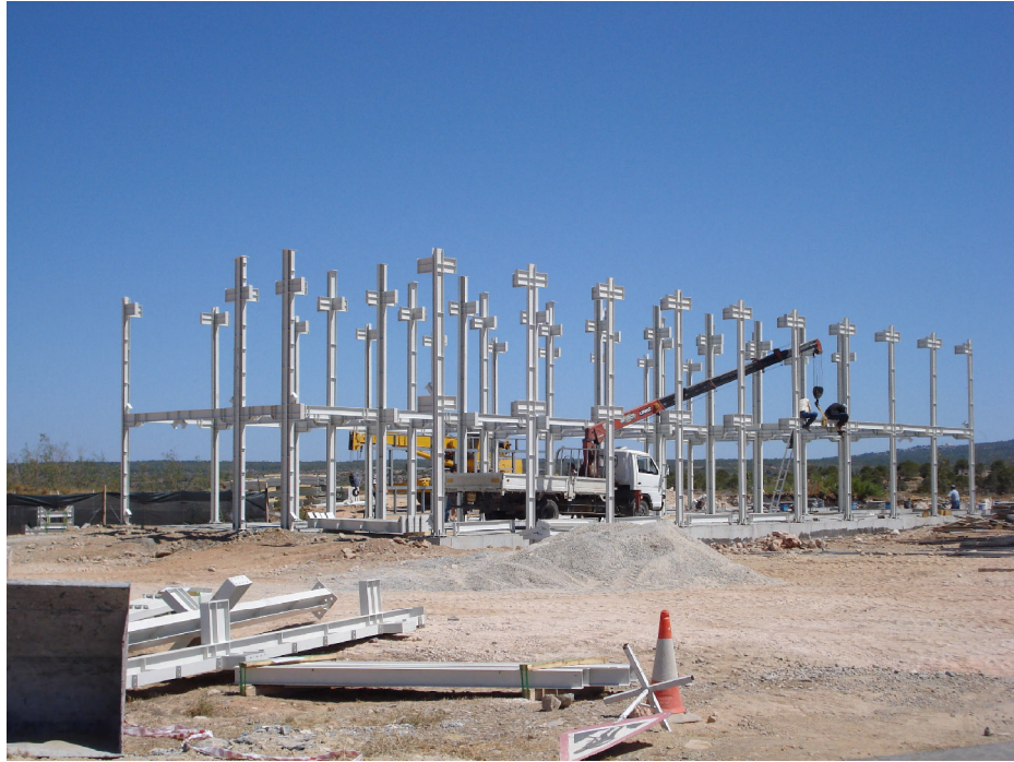
Figure 1.4: Flush end-plate splice connections used in a building frame (Turkish practice) (By courtesy of Caner)
