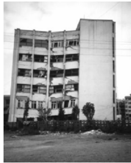
Figure 3.18 A Building Damaged due to Torsion Eccentricity 123
