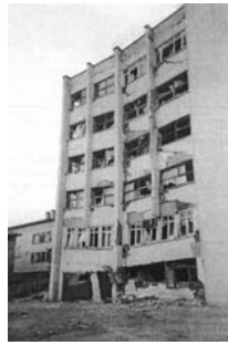
Figure 2.11 A Building Damaged due to Torsion Eccentricity 74
