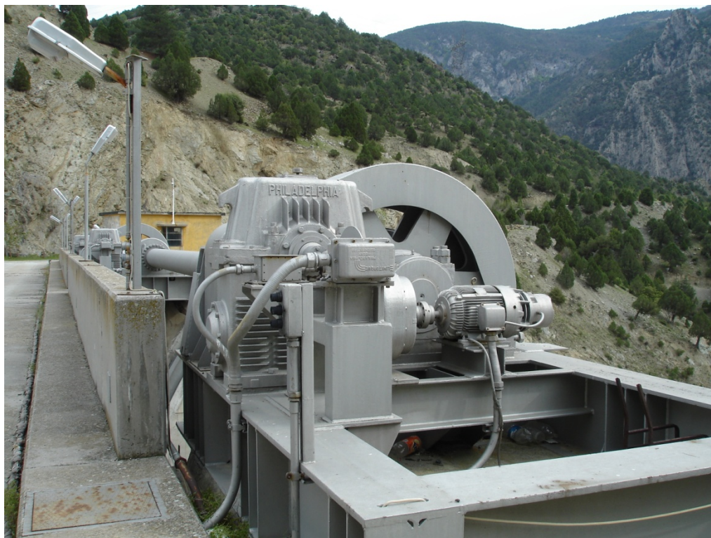
Figure 4.25 Spillway gate mechanism
