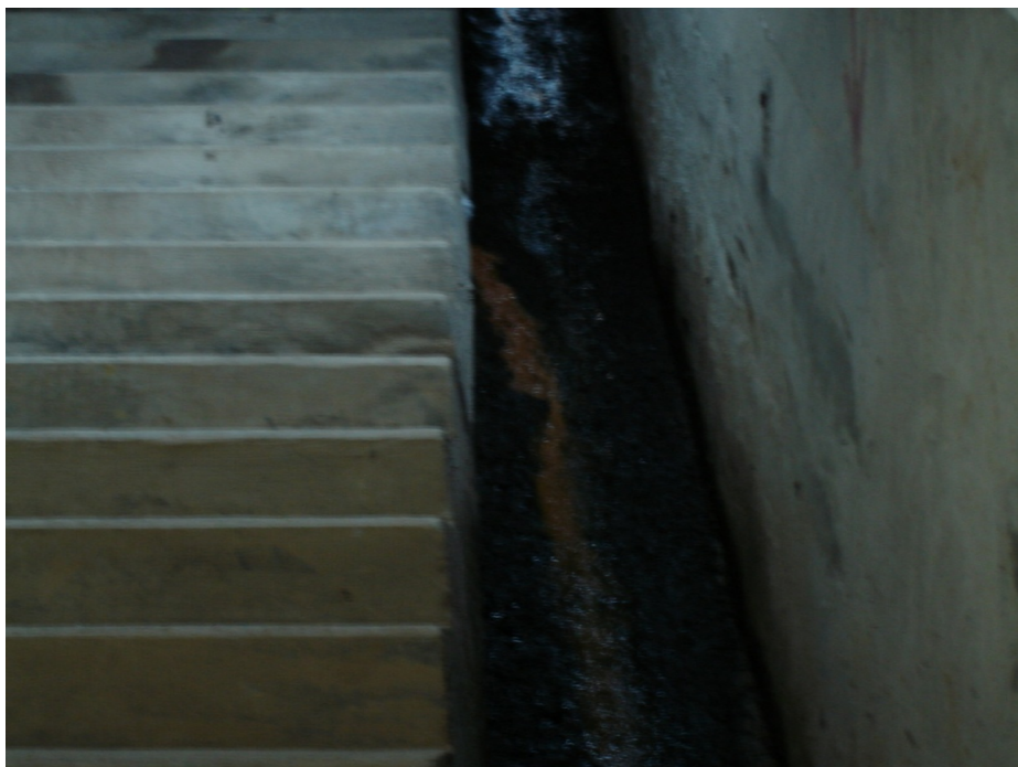
Figure 4.22 Traces of red mud in the drainage channel
