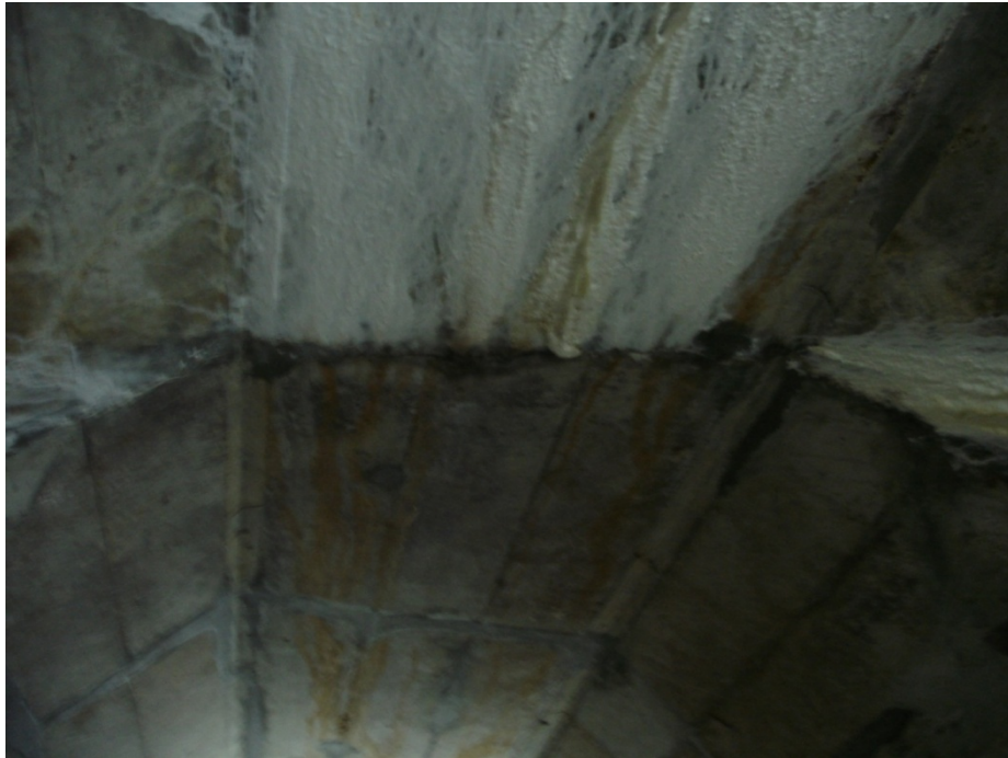
Figure 4.19 Calcium deposits at the ceiling of gallery
