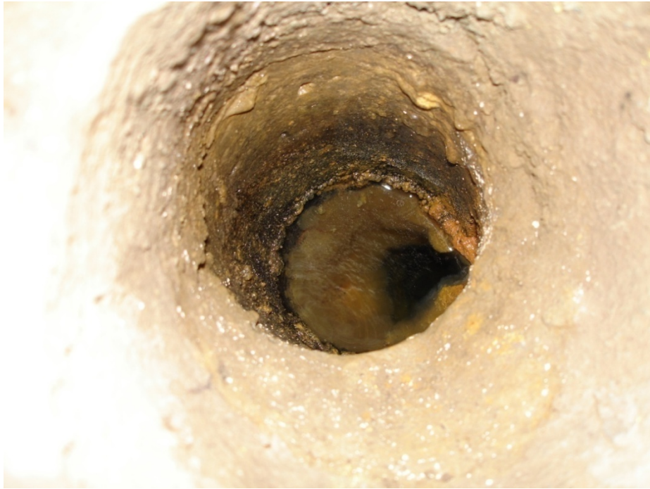
Figure 4.21 Red mud in a drain hole
