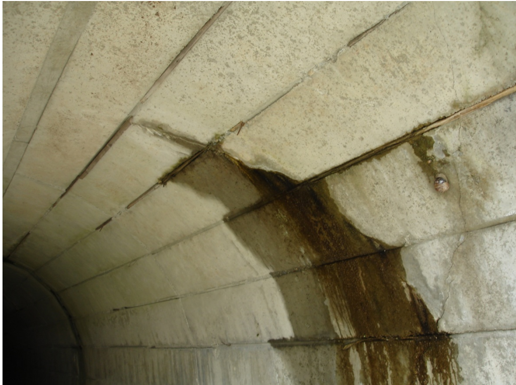
Figure 4.8 Seeping water through the ceiling of gallery
