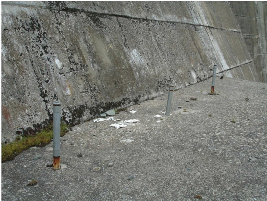
Figure 4.23 Standpipe piezometers on the right thrust block
