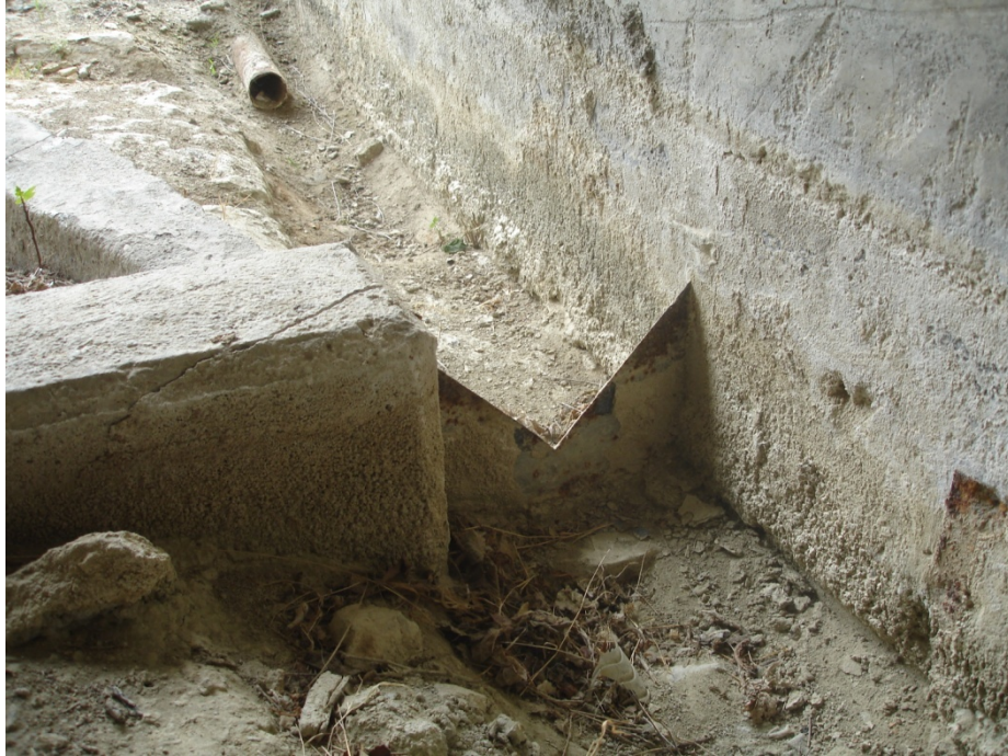
Figure 4.9 Accumulated debris at the weir
