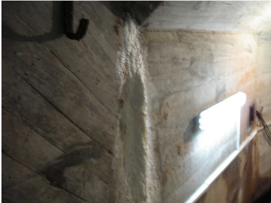
Figure 4.17 Calcium deposits along a construction joint
