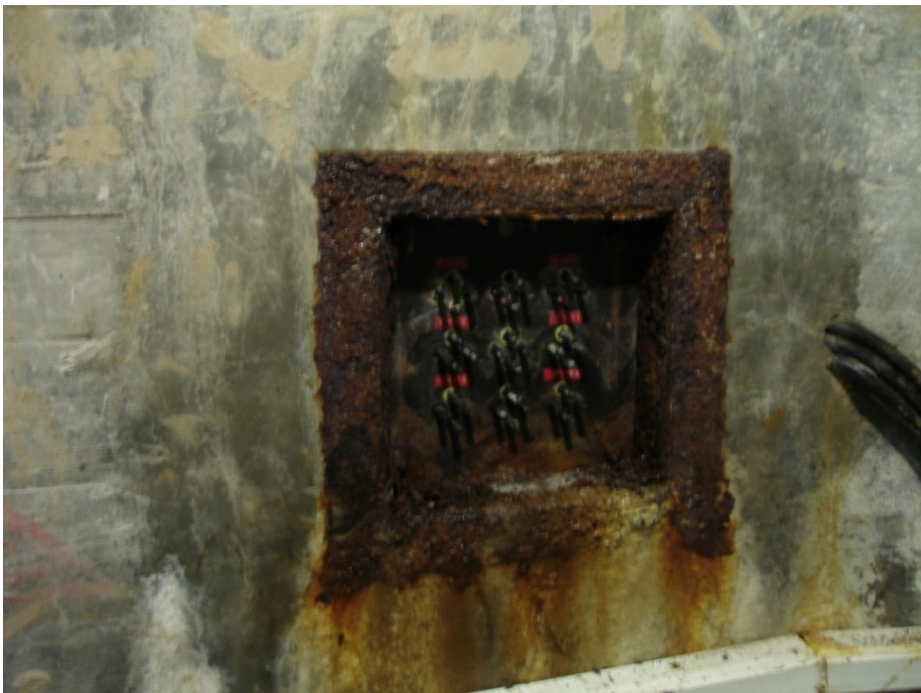
Figure 4.16 Corroded strainmeter ports
