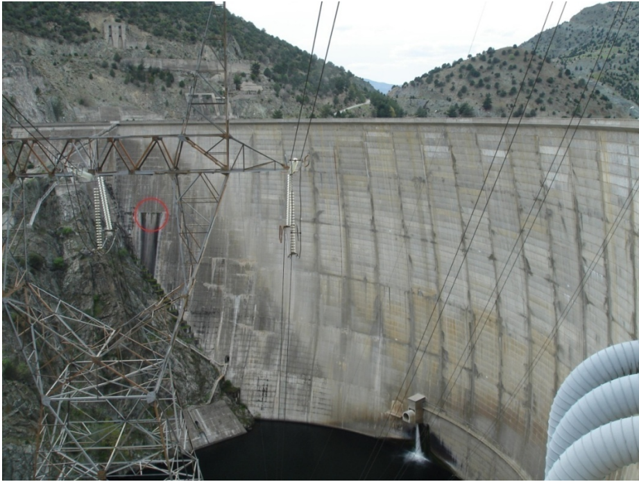
Figure 4.10 Crack on the face of the dam
