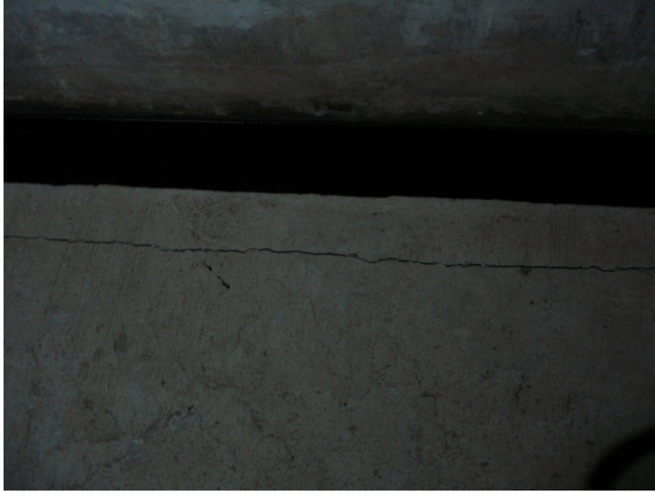
Figure 4.13 Crack on the base of the gallery
