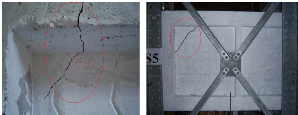
Figure 5.42 - Hairline Crack on the First Story Infill
