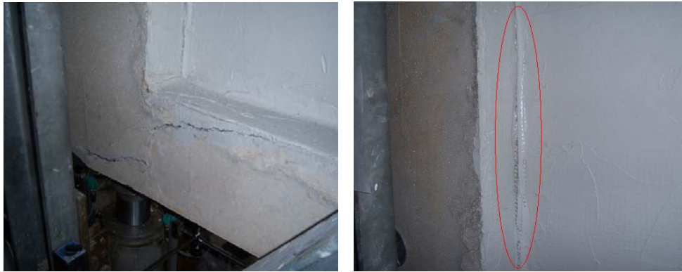
Figure A.6 - Column-Foundation Joint Crack (left) and Crack on the Infill (right)
