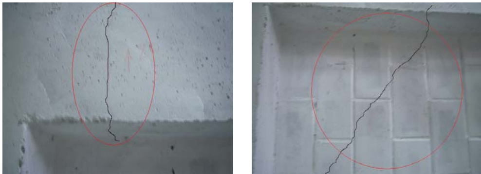
Figure 5.51 – Cracks on the Column (right) and on the First Story Infill Wall (left)
