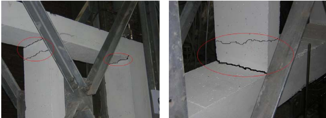
Figure 5.10 - Column-Beam Joint Cracks in the Fourth Cycle
