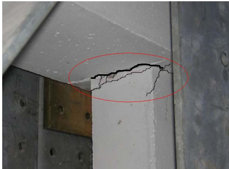
Figure 5.9 - Column-Beam Joint Crack at the Second Story Level
