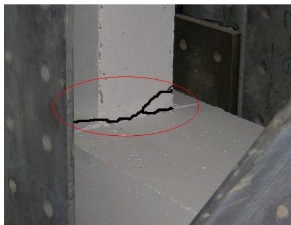
Figure 5.8 - Column-First Story Beam Joint Crack
