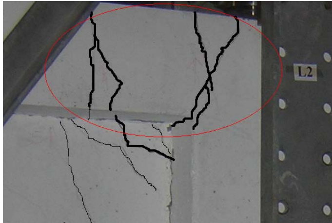
Figure 5.19 – Foundation Beam-Column Joint Cracks
