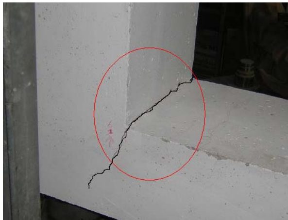
Figure 5.7 - Column-Foundation Joint Crack
