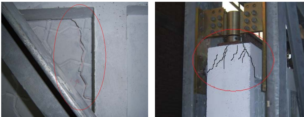
Figure 5.44 - Separation Between Blocks (left) and Cracks on the Support (right)
