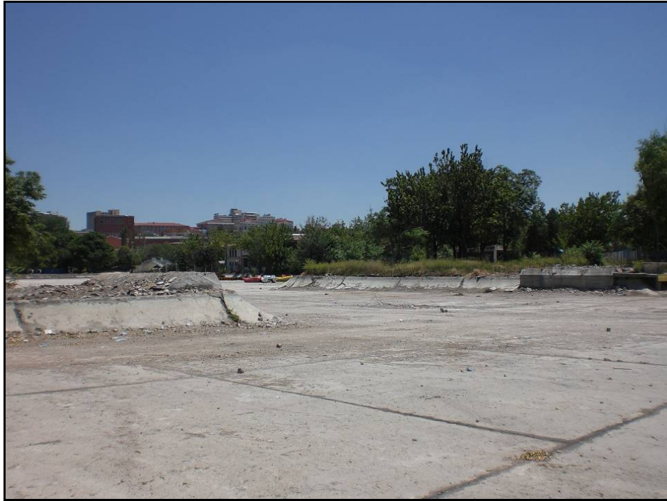
Figure 4.34 The Bridge in Gençlik Parkı; The Bridge after Demolition (Atilla Cangır, Cumhuriyetin Başkenti, no.617; Author, 18.06.2008)
