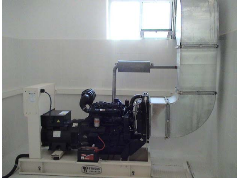
Figure IX.5. A view of the generator room
