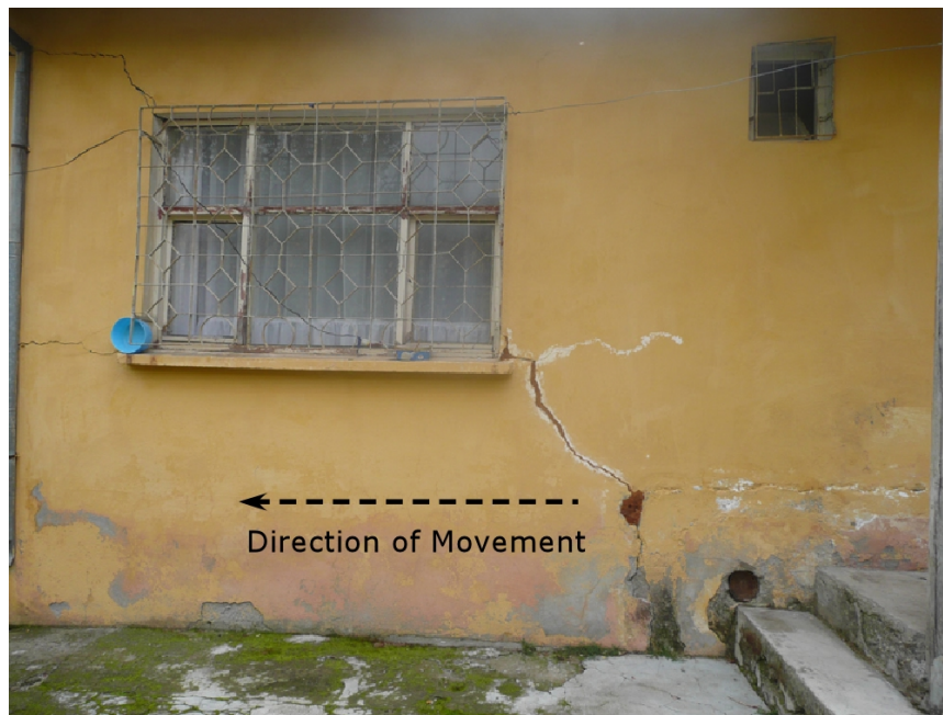
Figure 3.7 Cracks and fissures on the wall of house (photo taken from point f in Figure 4.1)
