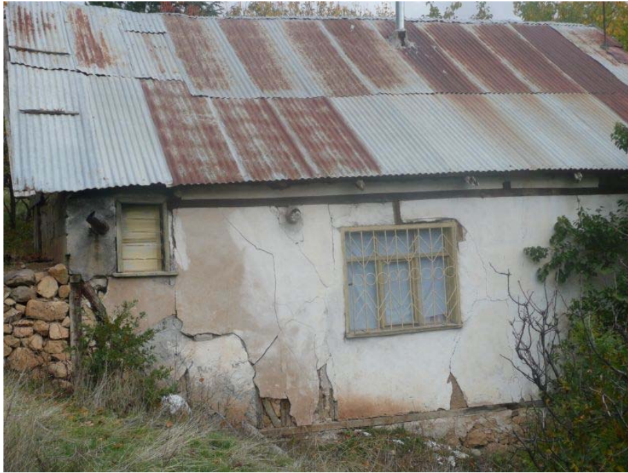
Figure 3.6. Cracks on the wall of house located at west of settlement area (photo taken from point e in Figure 4.1)
