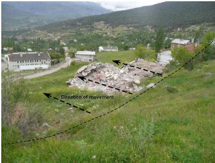
Figure 3.4. Ruined houses in the settlement area (photo taken from point c in Figure 4.1)
