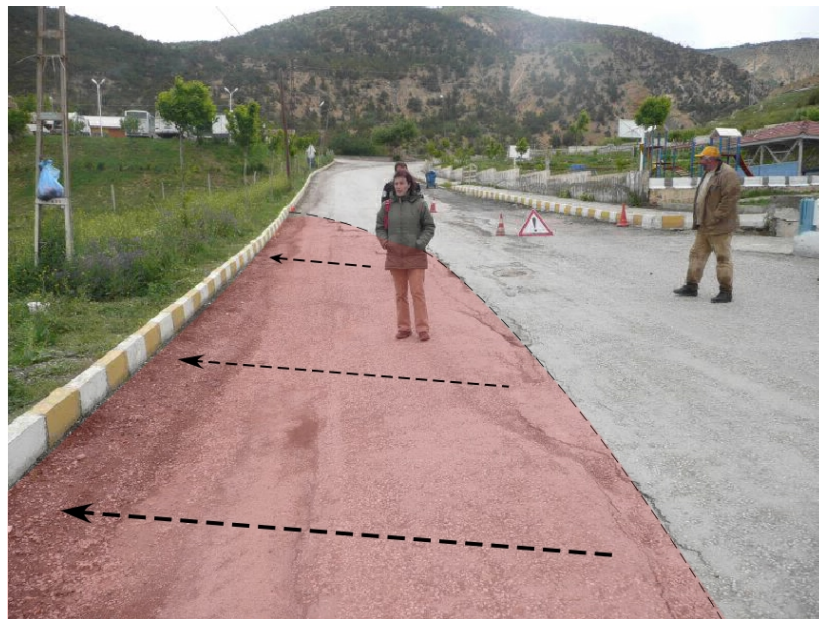
Figure 3.3. Deformed road moving toward south direction (photo taken from point b in Figure 4.1)
