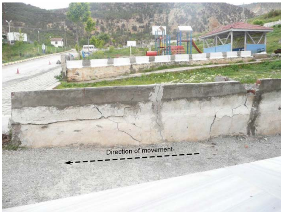
Figure 3.5. Cracks on wall near Police Station (photo taken from point d in Figure 4.1)
