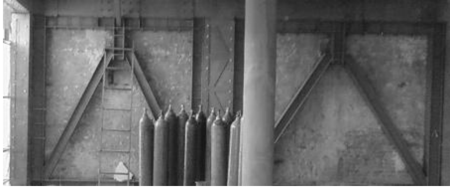
Figure 2.2 A recent application of the proposed retrofitting system to Halkbank Eskişehir branch office building
