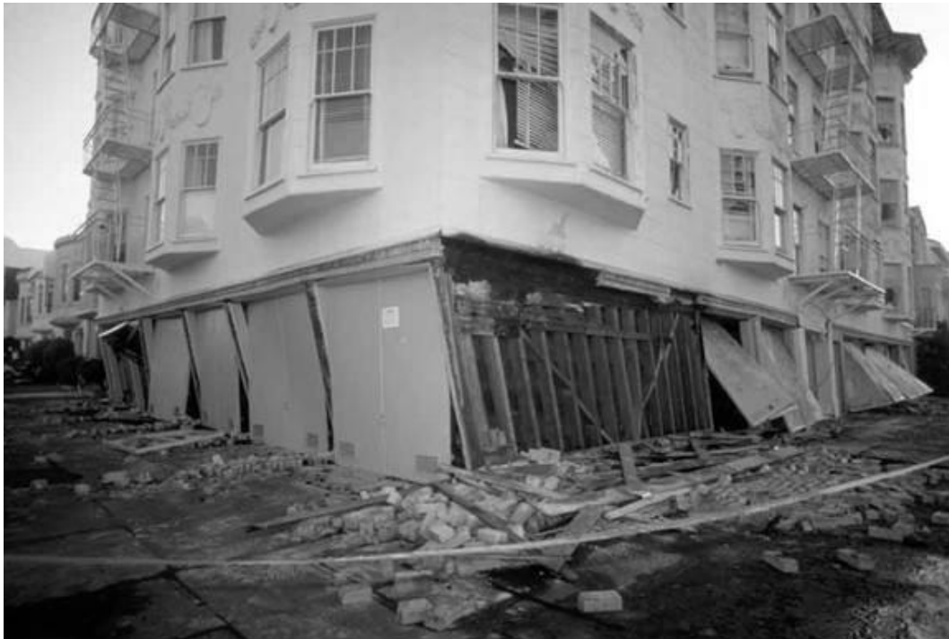
Figure 5.21 Soft story effect on a building (De Anza College Faculty Web Sites)
