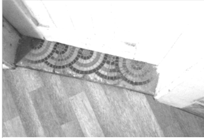
Figure 2.58: Detail of the floor at the threshold of the cellar source: (author, December 2008)
