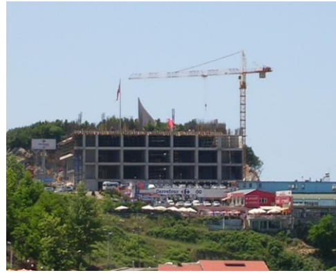
Figure 43. The construction area of Carrefour shopping mall Photograph by Şenay Işın, May, 2008
