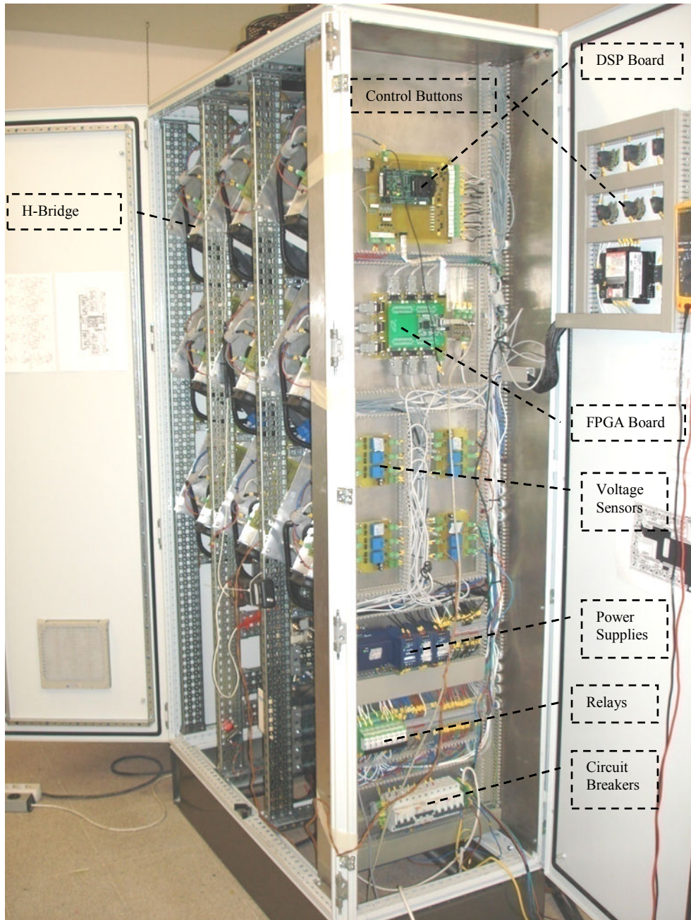
Figure 4.32 Side View of Enclosure, CMI Converter Stage and Control Stage
