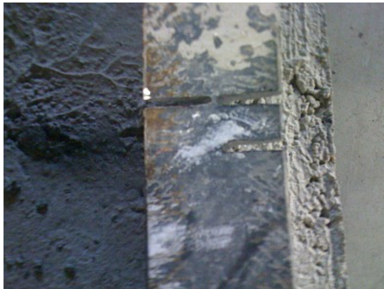
Figure B.3: Double Flange Cut (Damage Level 2)
