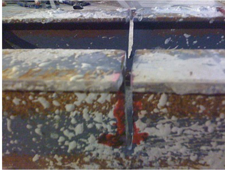
Figure B.6: Fourth Damage Level
