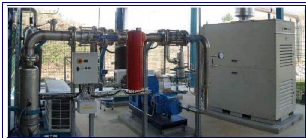
Figure 2.23 65 kW e Micro-turbine Co-generation Plant and Accessories installed (1 st Stage)
