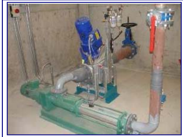
Figure 2.15 Reactor feeding pump and in-line macerator
