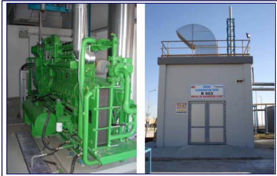
Figure 2.24 330 kW Gas Engine Co-generation Plant
