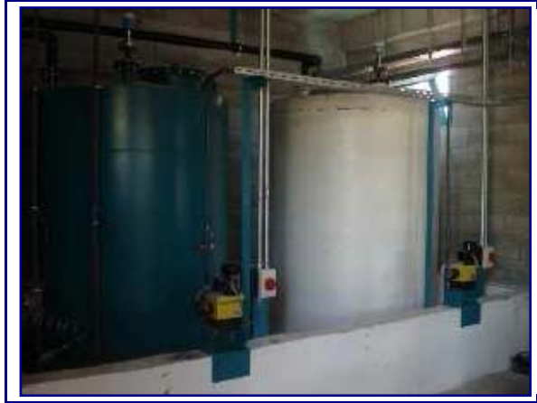
Figure 2.17 Chemical Dosing Station
