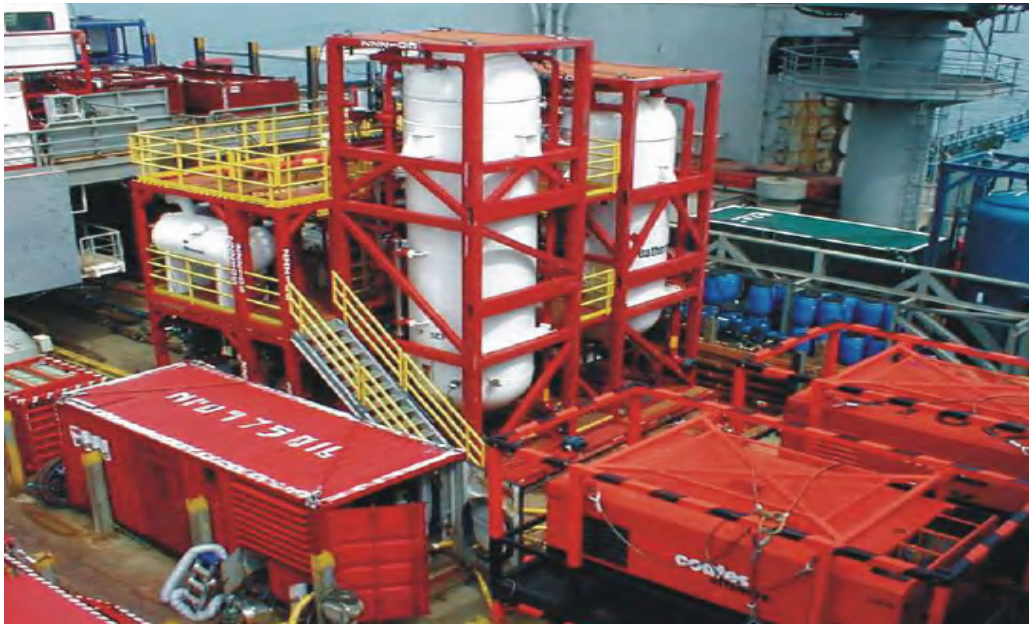
Figure 67 Multiphase Separation System for MPD 56
