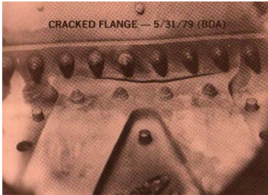
Figure 1.7 – A Cracked Flange of American Airplane [8]
