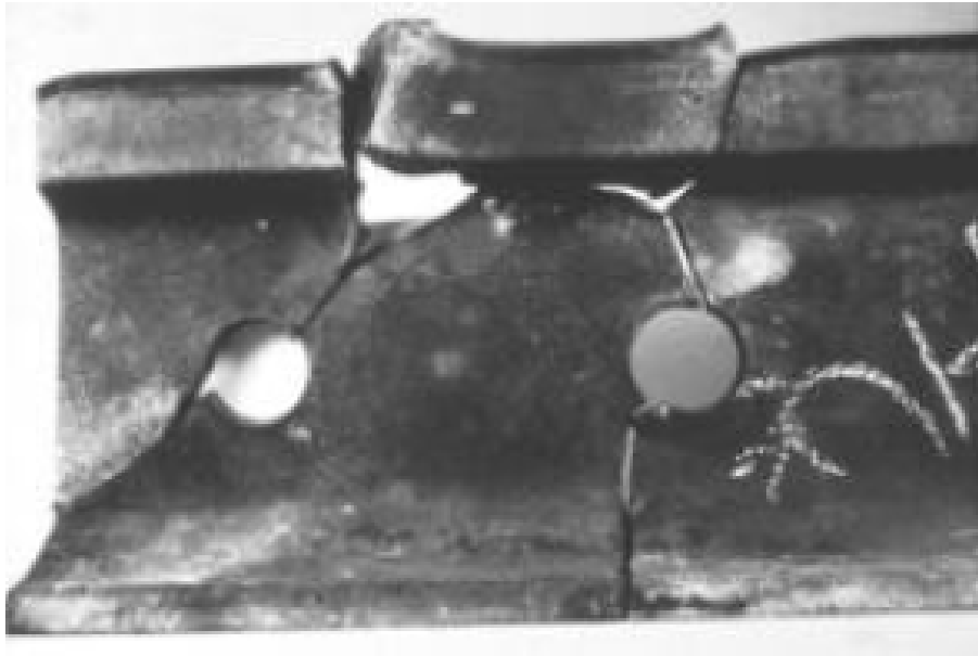
Figure 1.4 –Failure of a railway track component [52]
