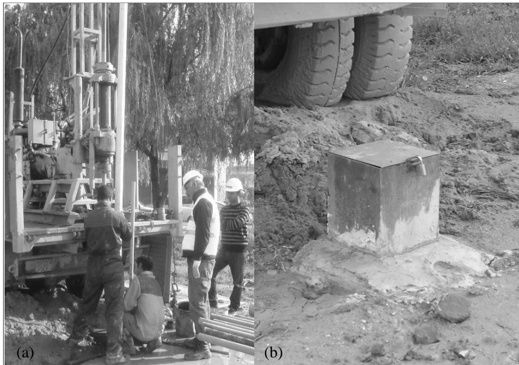
Figure 2.10 Preparation of the borehole for P-S suspension logging: a) installation of PVC pipes inside the borehole, b) the sealing of borehole.
