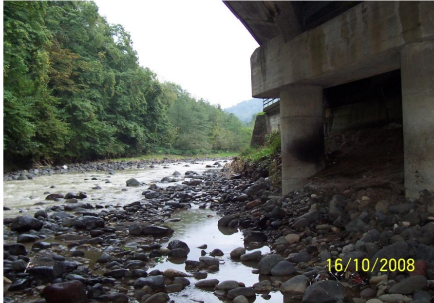
Figure 3.10 Mass wasting and aggradation in the upstream of Fol-1 Bridge
