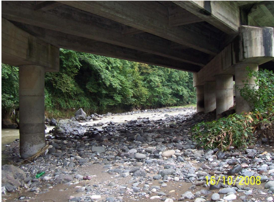
Figure 3.8 Excessive debris accumulations between piers
