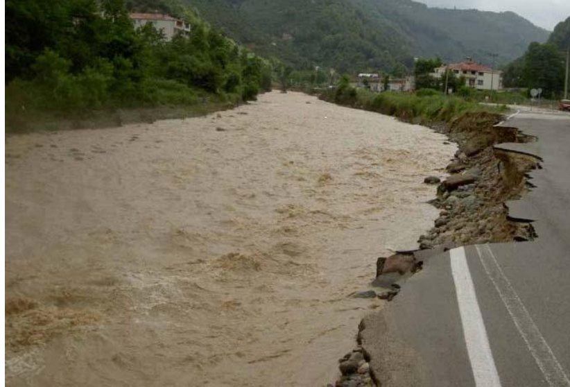
Figure 3.1 Highway is damaged due to flood (Tuna, 2008)
