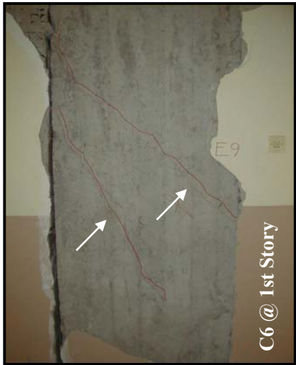
Figure 4.35 Shear cracks in the first floor column-C6 (Bolu)
