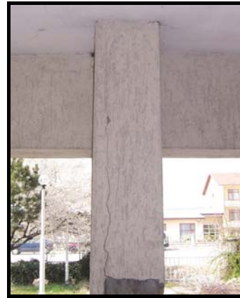
Figure 4.50 Exterior joint between the ground story column-C15 and beams B2-B3-B19 (Bolu)
