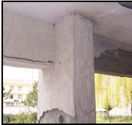
Figure 4.49 Exterior joint between the ground story column-C14 and beams B1-B2-B16 (Bolu)
