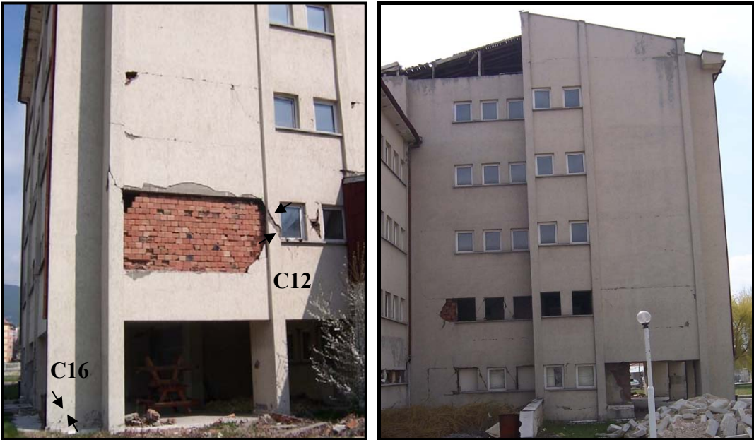
Figure 4.21 Lateral views from the Bolu building: Damage in infill walls, shear cracks in the ground story column-C16 and first story column-C12
