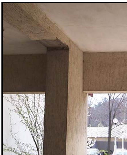
Figure 4.47 Exterior joint between the ground story column-C12 and beams B6-B22-B23 (Bolu)
