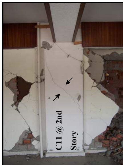
Figure 4.38 Shear cracks in the second story column-C11 (Bolu)
