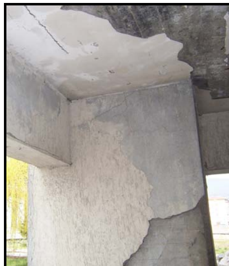
Figure 4.48 Corner joint between the ground story L-shaped column-C13 and beams B1-B13 (Bolu)
