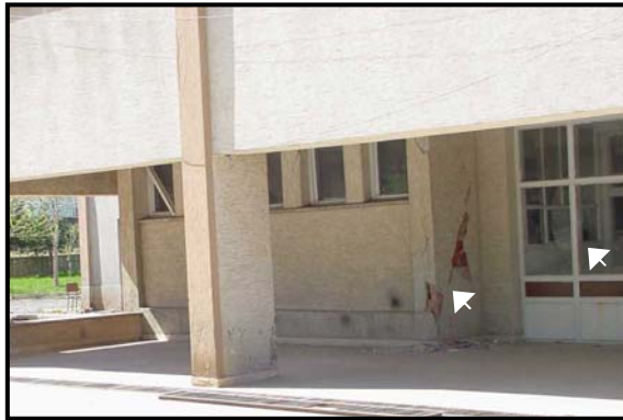
Figure 4.66 Structural damage to the ground story infill wall and broken windows (Bingöl)
