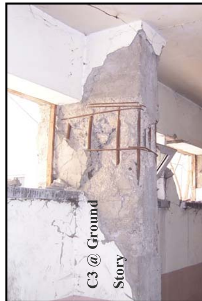
Figure 4.33 Damage to the ground story captive column-C3 (inside view)
