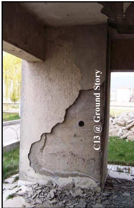
Figure 4.29 Shear cracks in the ground story column-C13 (Bolu)
