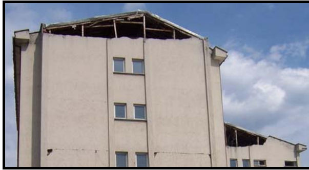
Figure 4.57 Damage to the roofs of the main and the adjacent building (Bolu)
