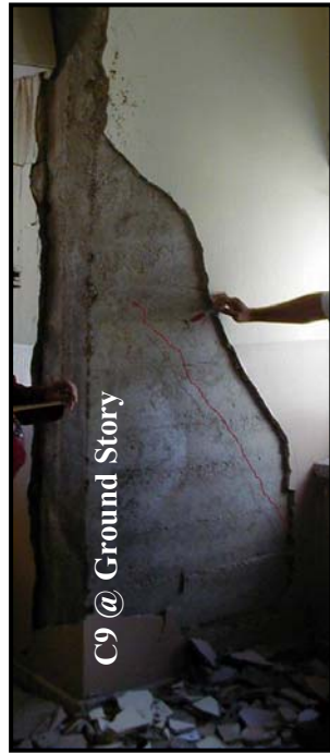
Figure 4.27 Shear cracks in the ground story column-C9 (Bolu)
