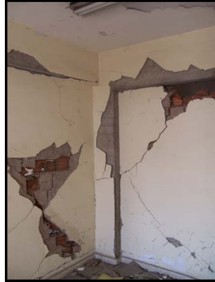
Figure 4.54 Severe damage to the infill wall in the first story (Bolu)
