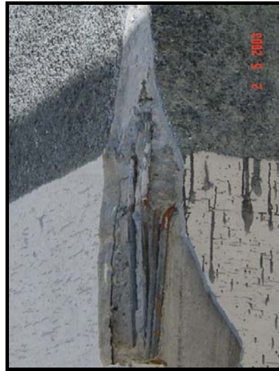
Figure 4.67 Disengagement of reinforcement bars in the columns (Bingöl)
