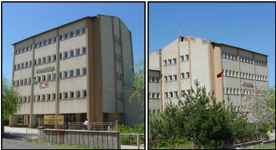
Figure 4.60 Side views of the MPWR building in Bingöl after the 2003 earthquake (a) the case study building, (b) the case study building and the adjacent four-story facility
