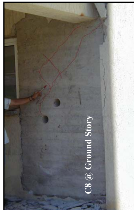
Figure 4.26 Shear cracks in the ground story column-C8 (Bolu)
