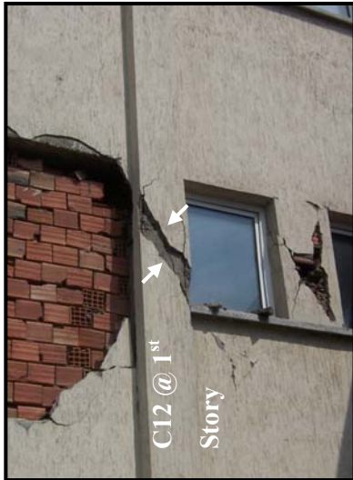
Figure 4.36 Shear cracks in the first story column-C12 (Bolu)
