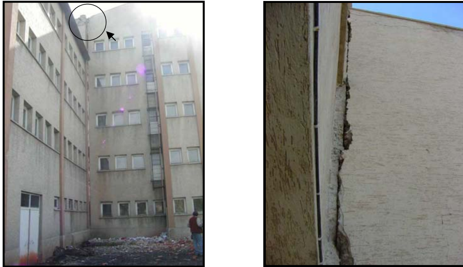
Figure 4.61 Impact was observed at the roof with the adjacent mid-rise building (Bingöl)
