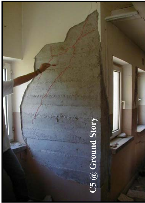
Figure 4.23 Shear cracks in the ground story column-C5 (Bolu)
