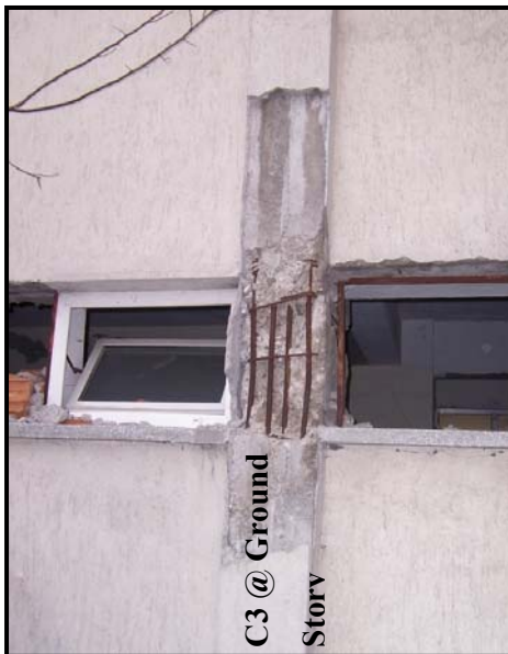
Figure 4.32 Damage to the ground story captive column-C3 (outside view)
