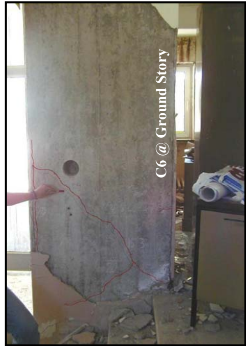
Figure 4.24 Shear cracks in the ground story column-C6 (Bolu)
