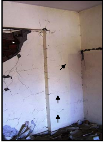
Figure 4.39 Shear and flexural cracks in the second story column-C12 (Bolu)
