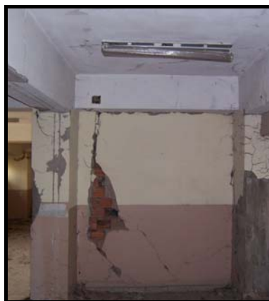
Figure 4.51 Severe damage to the infill wall between the ground floor columns-C6 and C10 (Bolu)
