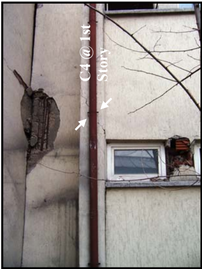
Figure 4.34 Shear cracks in the first story L-shaped corner column-C4 (Bolu)
