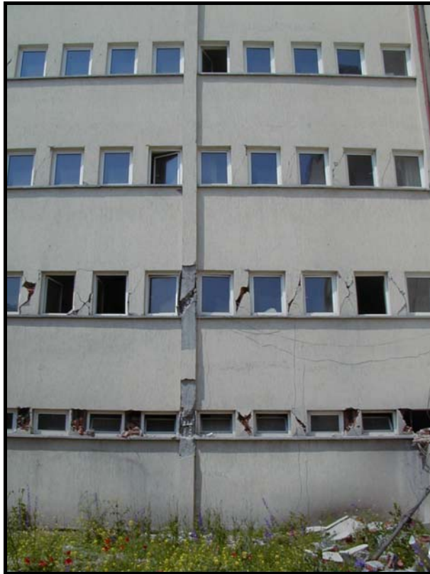
Figure 4.20 Rear view of the Bolu building: Infill failures at the bottom three stories and shear failures of the captive columns at the ground and first story
