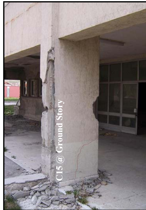
Figure 4.30 Shear cracks in the ground story column-C15 (Bolu)
