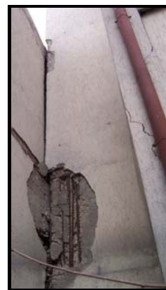
Figure 4.59 Longitudinal reinforcement in the first story L-shaped corner column-C4
