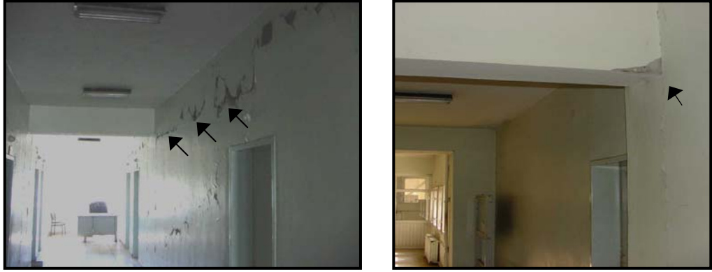
Figure 4.65 Light damage to the beams (Bingöl)
