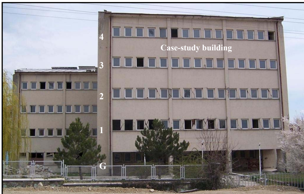
Figure 4.19 (a) Front view of the Bolu building: Shear failures in masonry infills between the narrow windows
