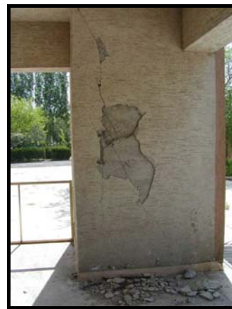
Figure 4.64 Extensive shear crack in the ground floor L-shaped column-C16
