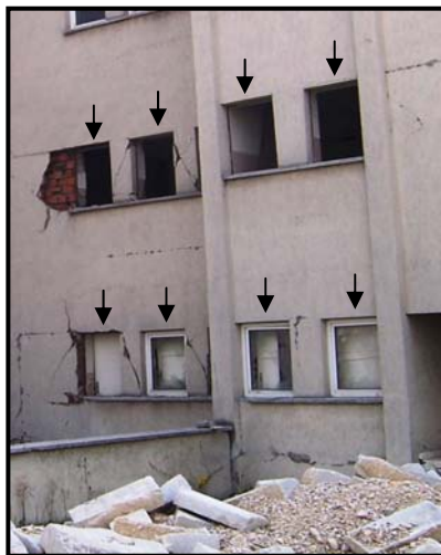
Figure 4.55 Nonstructural damage: The broken windows (Bolu)
