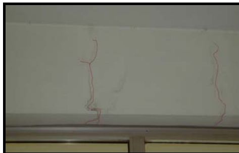
Figure 4.41 Flexural cracks in the ground floor beam-B8 (Bolu)
