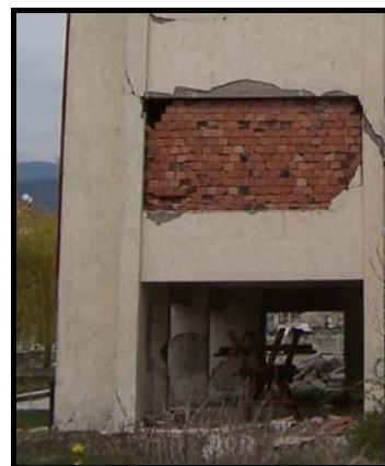
Figure 4.52 Severe damage to the infill wall between the first floor columns-C12 and C16 (Bolu)
