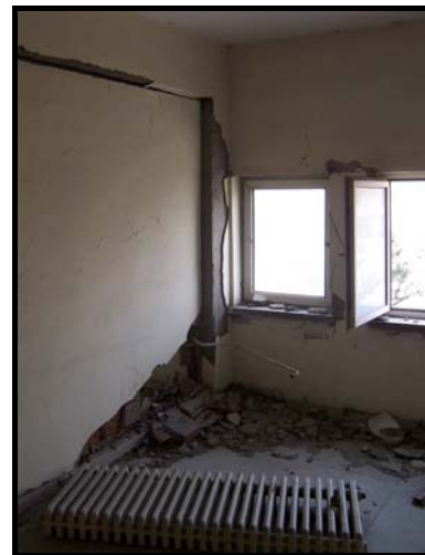
Figure 4.56 Nonstructural damage to the heating system and partition walls (Bolu)
