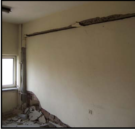
Figure 4.53 Severe damage to the infill wall between the first floor columns-C11 and C15 (Bolu)
