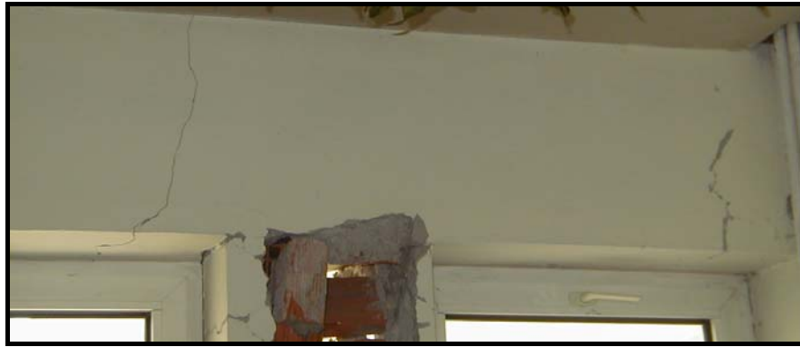
Figure 4.42 Flexural cracks in the ground floor beam-B12 (Bolu)
