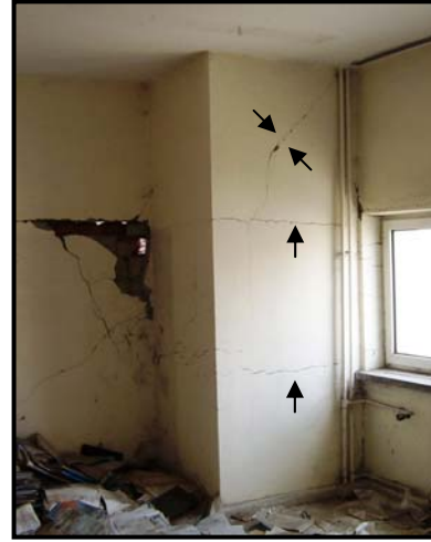
Figure 4.40 Shear and flexural cracks in the second story L-shaped corner column-C16
