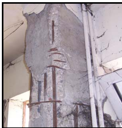
Figure 4.58 Disengagement of ties (Bolu)
