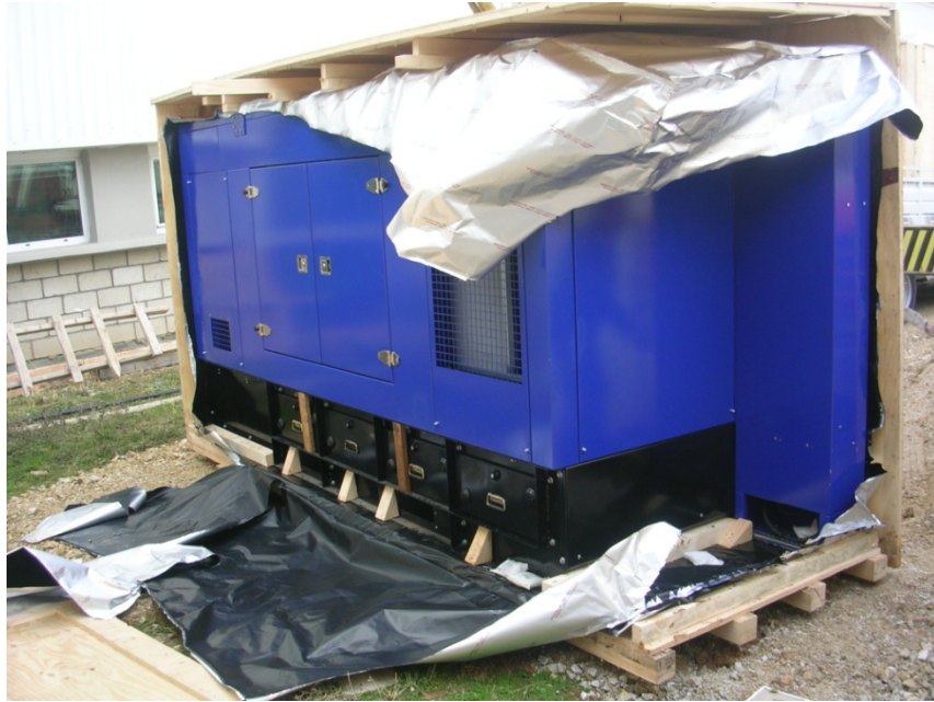
Figure D.3 Unwrapping the ICE Co-generator
