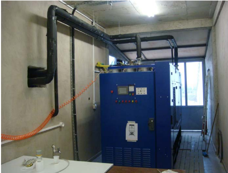
Figure D.8 ICE After the Construction- Inside the HEGEL Room
