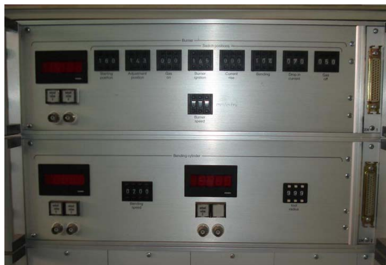
Figure 18 Electronic Control Unit of the MVT Equipment
