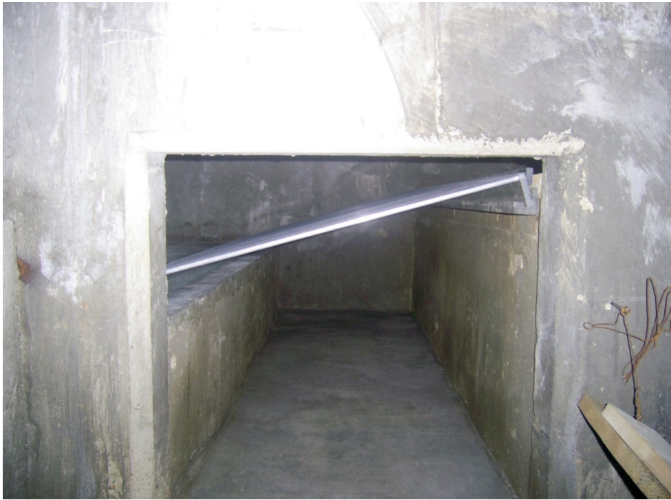
Figure 3.4 Side view of the trash rack and the collection channel
