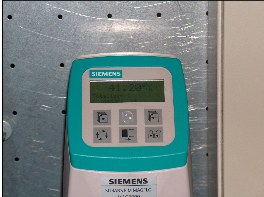
Figure 6.12 Manually Recording Discharge Values from Flowmeter's Panel during Step Test
