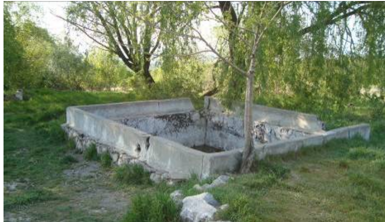
Figure 4.30. Idle concrete structure in the Yalıncağ Area
