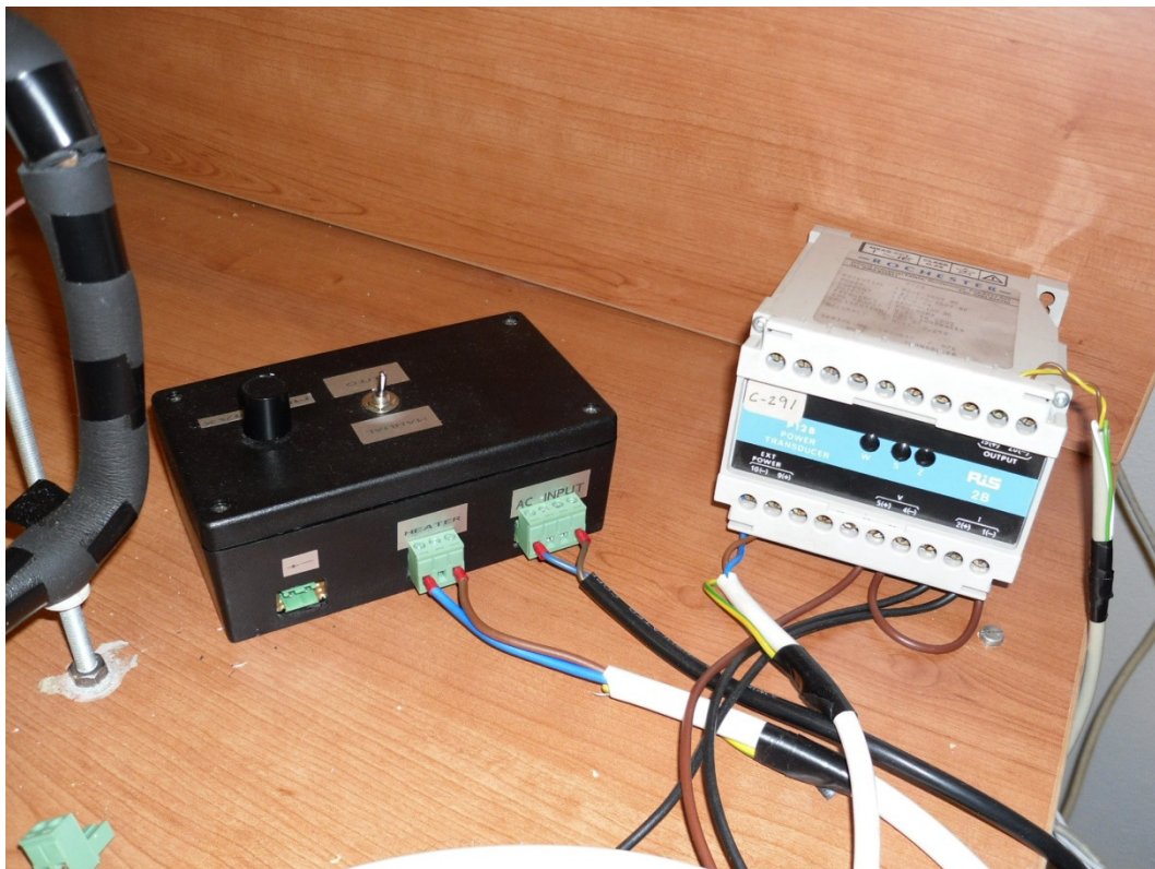
Figure 13: The control box and the power transducer of the pre-heater
