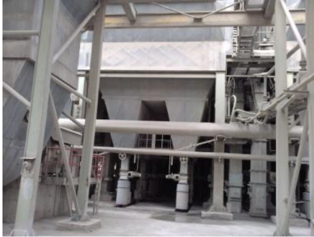
Figure 2.3 A photo from electrostatic precipitators of Soma Thermal Plant
