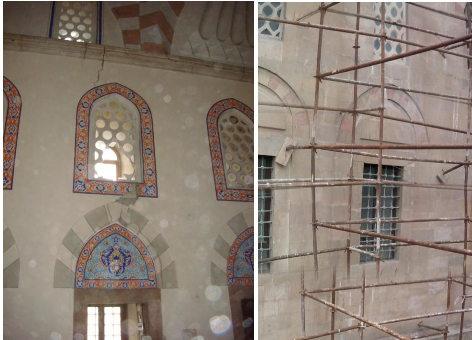
Figure 4.31 The cracked section of the wall
