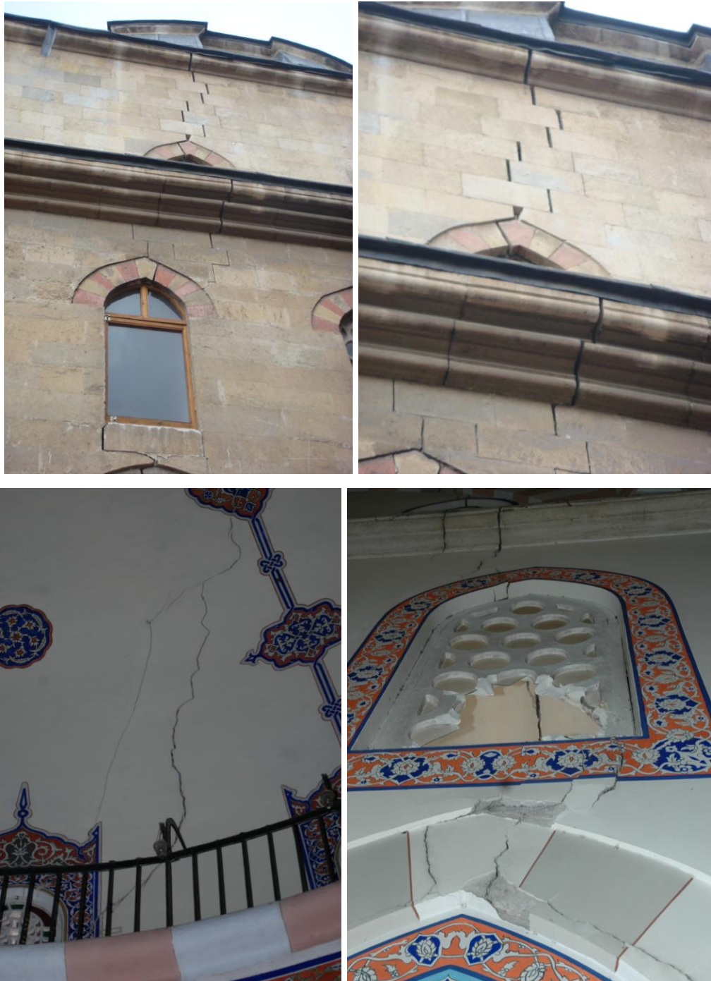
Figure 4.13 General views of cracks
