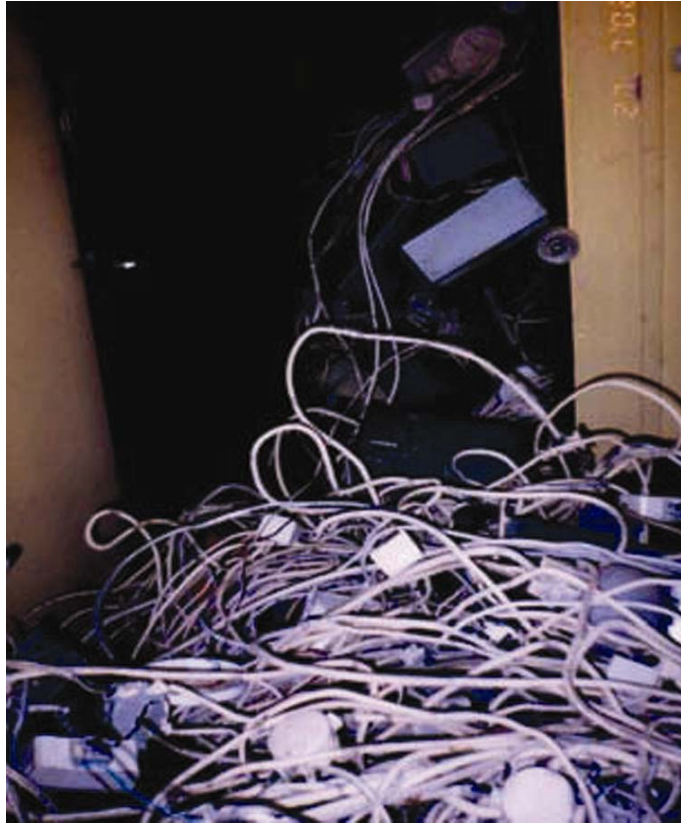
Figure 49 Inappropriate storage of electrical materials of prefabricated houses.
