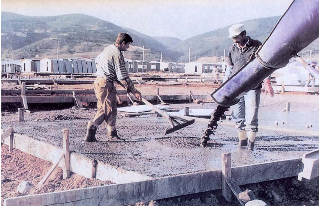
Figure 46 The construction of concrete basement of prefabricated temporary houses in settlements in 1999.
