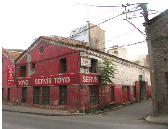
Figure B-13 A Warehouse in Alsancak in Darelict Condition
